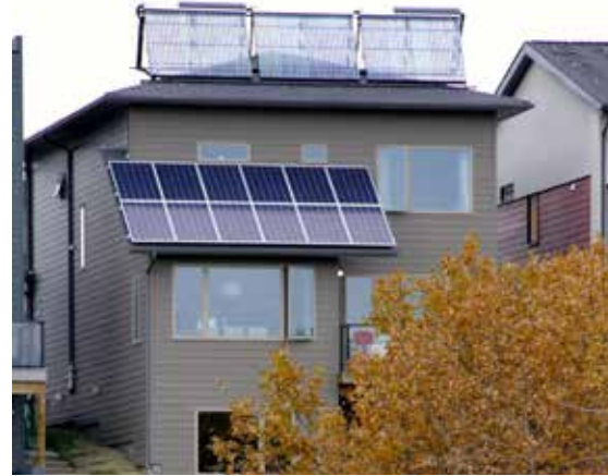
Solar thermal heating and solar photovoltaic panels. Photo credit: David Dodge, GreenEnergyFutures.ca
