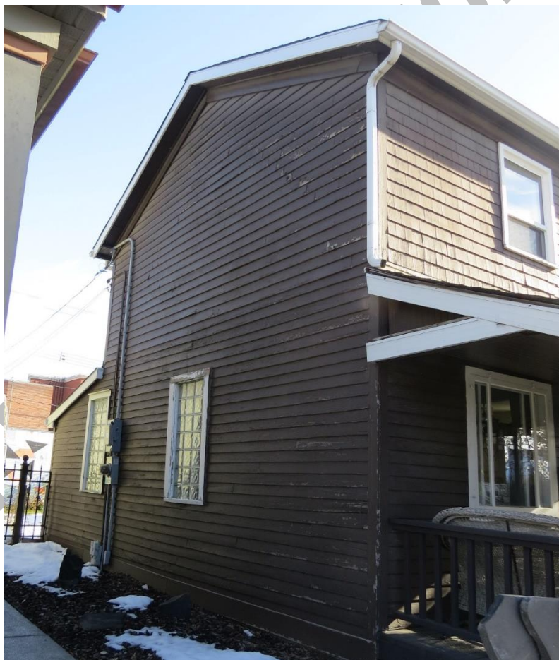
(Image 2.10 – South and west façades, showing beveled wood siding, and wood shingle cladding on south façade second storey)
