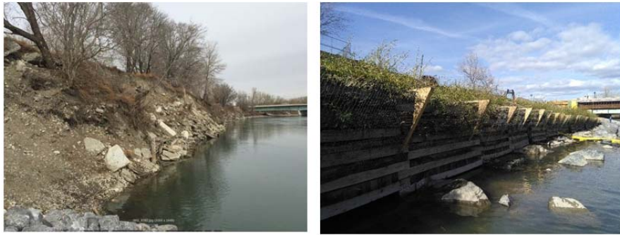
FIGURE 4.12 THE BIOENGINEERING DEMONSTRATION AND EDUCATION PROJECT SITE 1 BEFORE (LEFT) AND AFTER (RIGHT). (PHOTO CREDIT (RIGHT): KERR WOOD LEIDAL)
