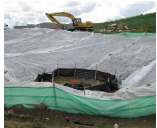
FIGURE 4.9 EROSION AND SEDIMENT CONTROL DURING CONSTRUCTION HELPS PROTECT THE WATERSHED AND STORM INFRASTRUCTURE.
