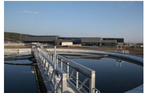
FIGURE 4.2 PINE CREEK WASTEWATER TREATMENT PLANT
