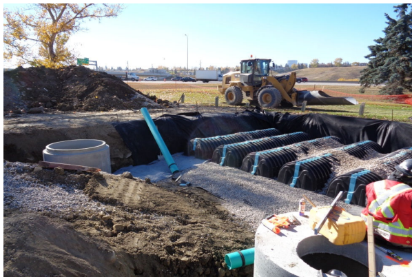
Deerfoot Athletic Park rain garden and infiltration chamber
