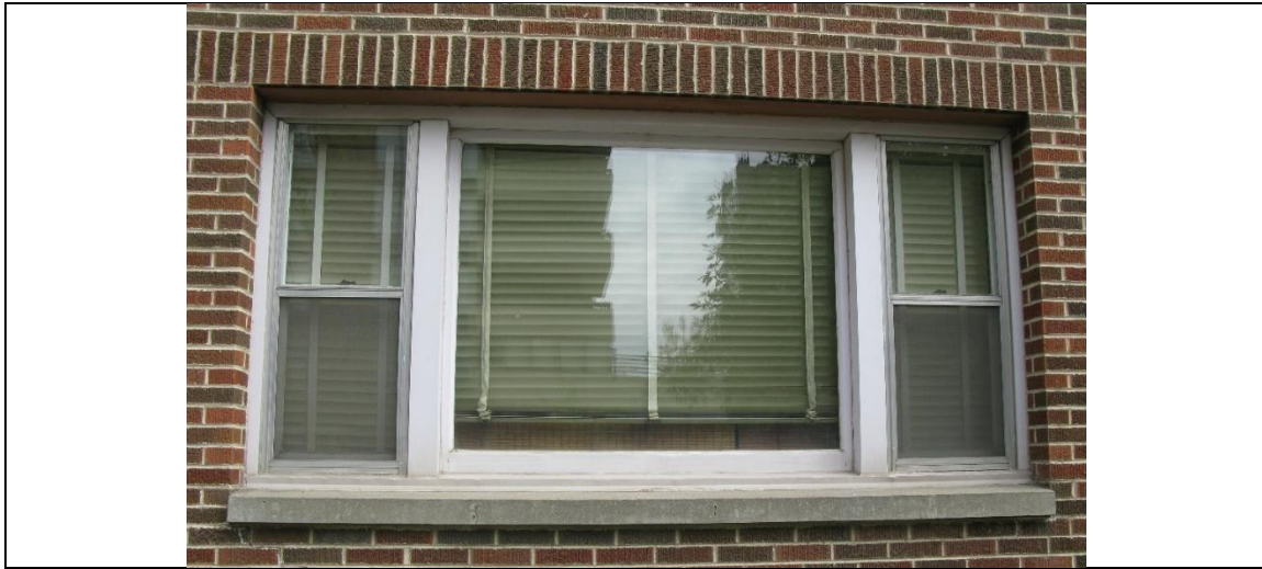
(Image 1.9: example of triple assembly wooden frame windows with one-over-one profiles flanking a fixed sash; concrete window sill)
