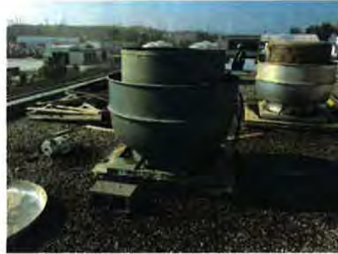
Photo 2 – Scalding: Odour sample collected from the exhaust of one of two identical roof fan units. The sample tube was inserted approximately 10-15 cm below the top of the exhaust rim mid-way between the center cap and the outer rim.
