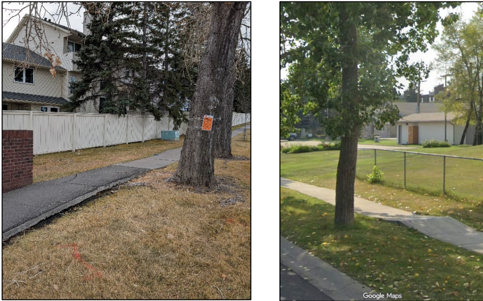
Figure 1: Sidewalk heaving damage due to the proximity of a shallow root system. This type of sidewalk damage is observed through many established communities across Calgary.
