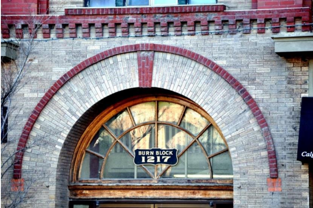
(Image 3.6: Detail of double brick arch above central main entry with upper arch and keystone detail made with red-coloured rusticated brick and the lower arch with buff-coloured brick in a radiating voussoir and wood half-round transom window)
