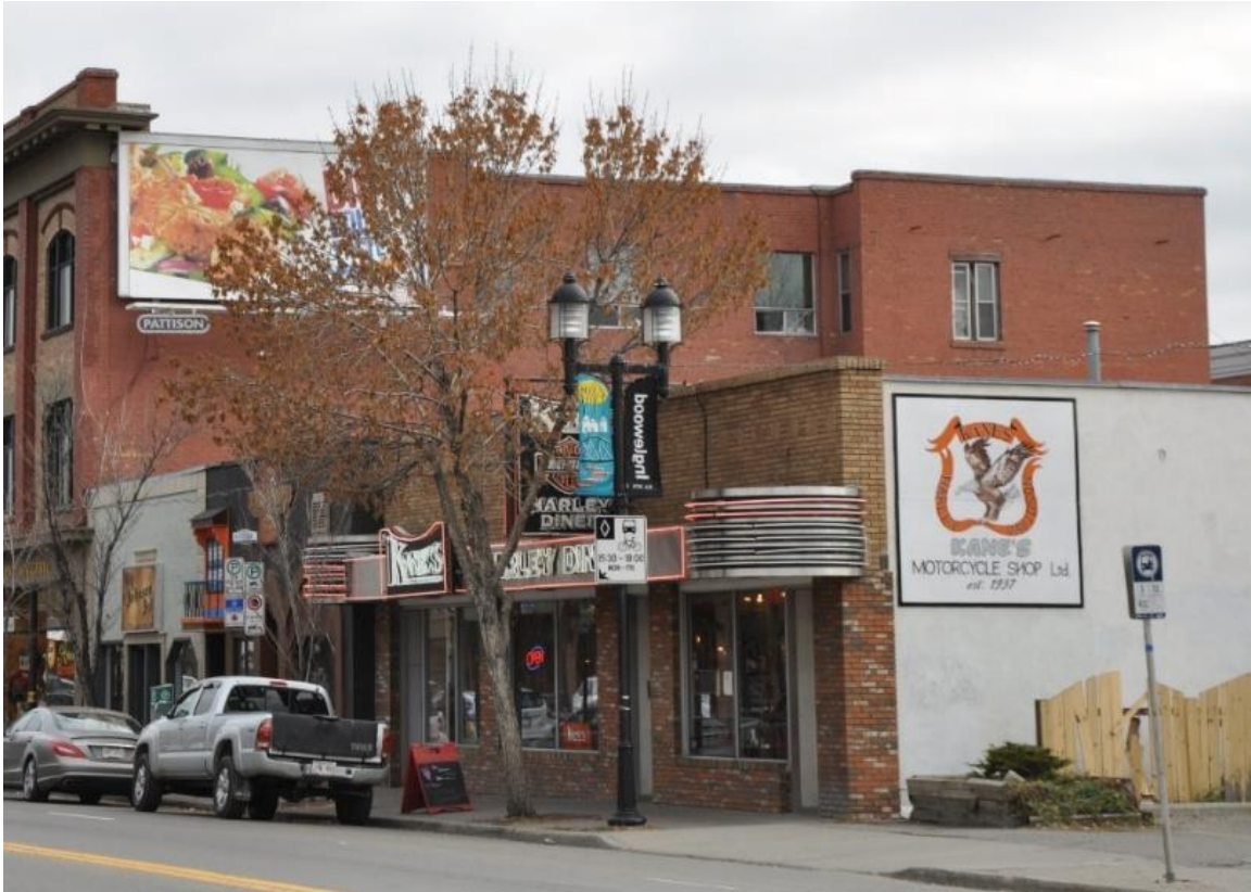
(Image 4.1: Oblique view of west façade showing brick cladding, parapet edge and light well)
