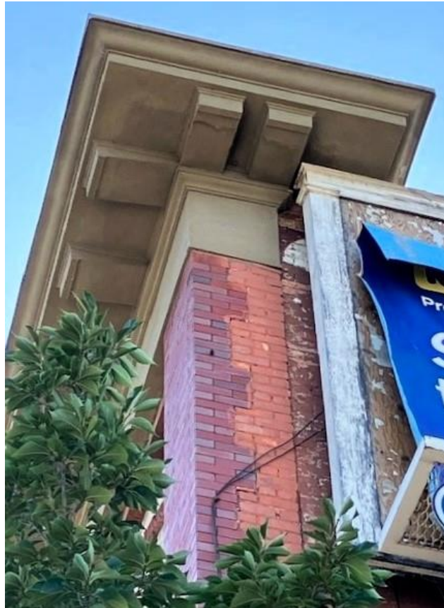
(Image 3.5: Detail of pressed metal upper cornice with dentils that wraps around the front corner of the side façade.)
