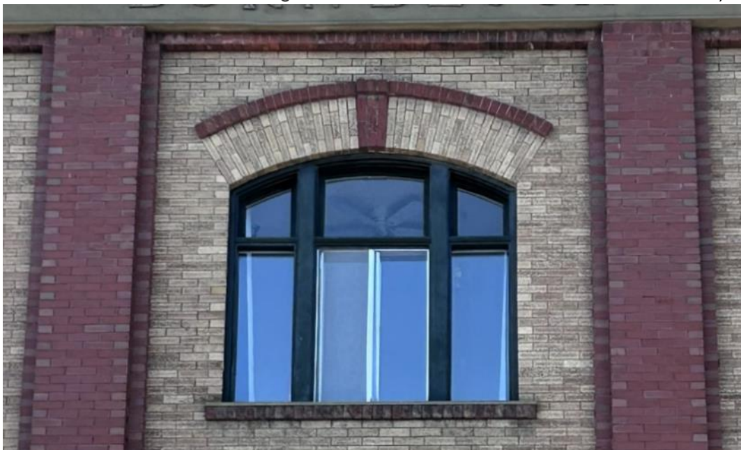
(Image 3.7: Example of fenestration on third storey of the north façade showing segmental arch lintel comprised of red-coloured brick in rowlock course with brick keystone, buff-coloured brick in a radiating voussoir and sills made up of brown-coloured brick in rowlock course. Note: the red coloured, smooth faced and buff-coloured, speckled brick cladding is laid in courses simulating quoins to add aesthetic detail to the pilaster and window frame edges)
