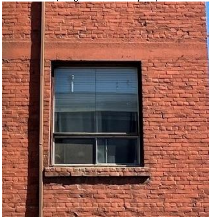
(Image 5.2: Detail of brick cladding in common bond pattern and example of sills made up of a header course and a stretcher course)
