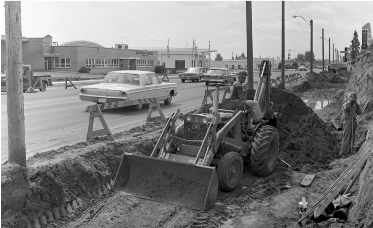
Macleod Trail widening project to expand from 4 to 6 lanes in 1966. Courtesy of Glenbow Archives.
