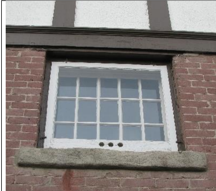
(Image 2.4: example of one of two 15-pane wood windows with concrete sills; continuous wood band with decorative trim)
