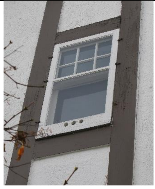
(Image 2.5: example of one of three 6-over-1 wood hung windows with flat heads and painted wood trim)
