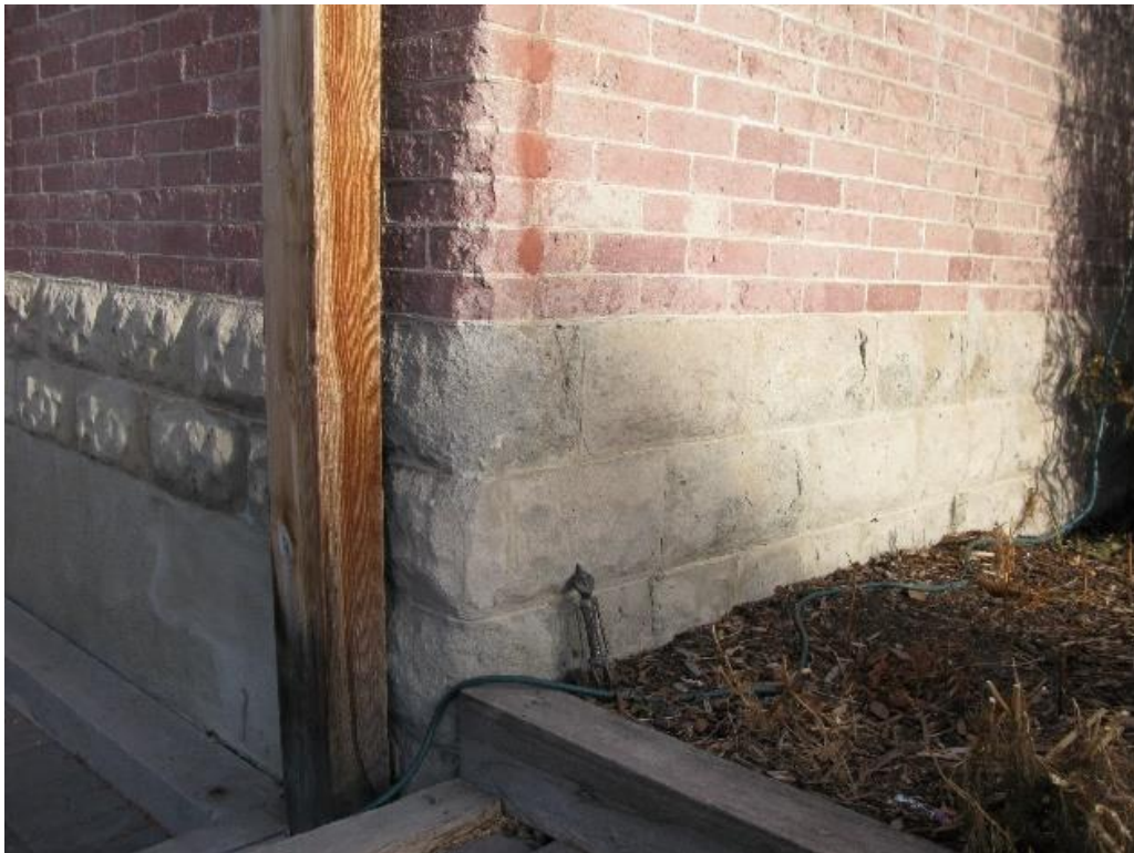
(Image 1.3 Stretcher bond concrete brick cladding; continuous hollow rock-faced concrete block band (three rows in south-facing façade, transitioning to two rows))
