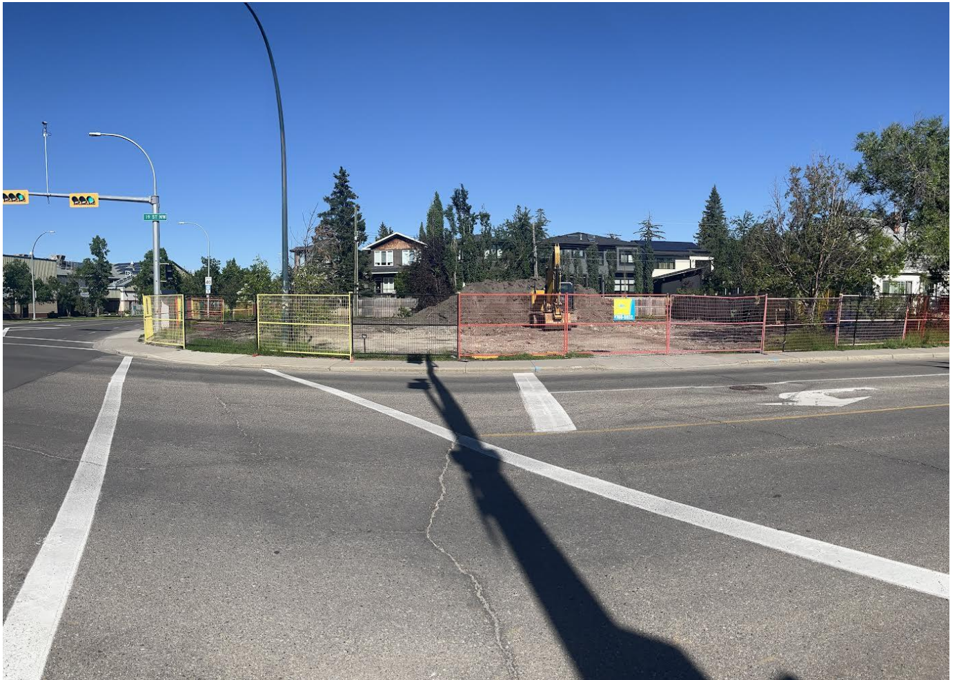
View from 19 th Street NW and 6 th Avenue NW - looking east to 526 & 530 19 th Street development
