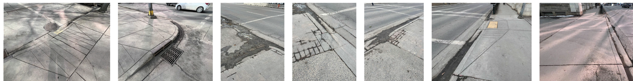
21 SITE PHOTO VIEW OF CURB CUT AT NORTH WEST OF SITE NTS 20 SITE PHOTO VIEW OF CATCH BASIN AT NORTH WEST OF SITE NTS 19 SITE PHOTO VIEW OF CURB CUT NORTH OF CALLAGHY PUBLIC BUILDING NTS 18 SITE PHOTO VIEW OF CURB CUT AT 8 AVENUE SE NTS 17 SITE PHOTO VIEW OF CURB CUT AT 8 AVENUE SE NTS 16 SITE PHOTO VIEW OF CURB CUT SOUTH OF DOMINION BANK BUILDINGS NTS 15 SITE PHOTO VIEW OF CURB CUT AT DOMINION BANK BUILDINGS NORTH LANE NTS
