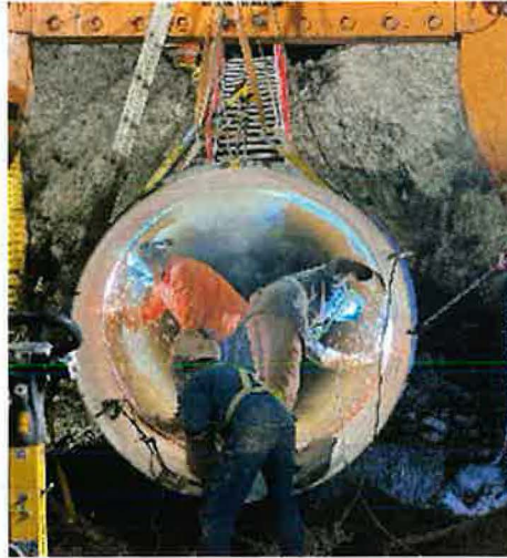
Aging, critical infrastructure
