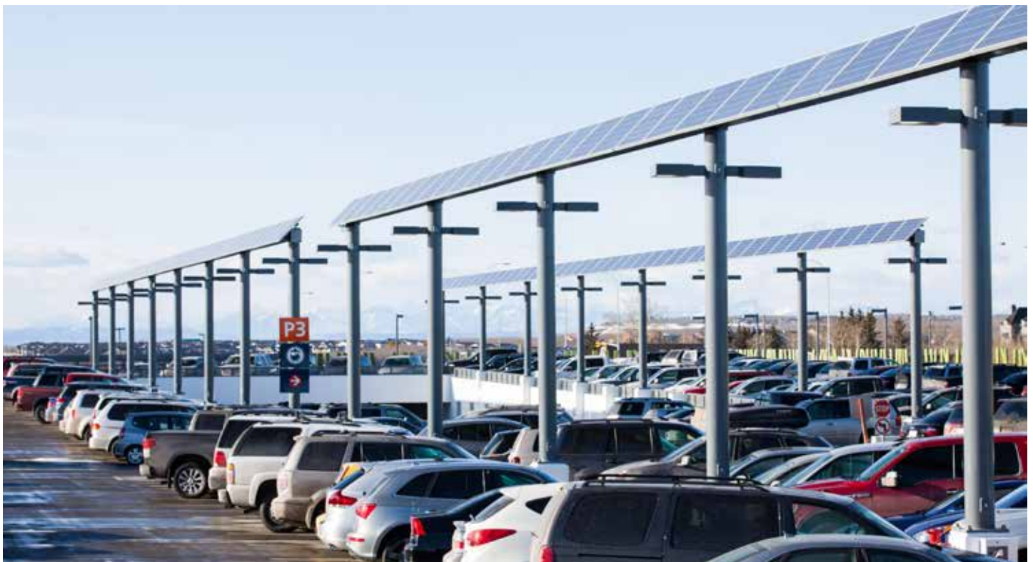
Solar installation at the 69th Street Station Park and Ride. ISC: Unrestricted
