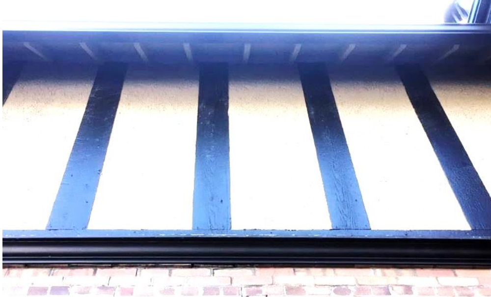
(Image 3.6: Close up of moulded wood cornice above brick cladding, decorative wood half-timbering and eaves with exposed rafters)
