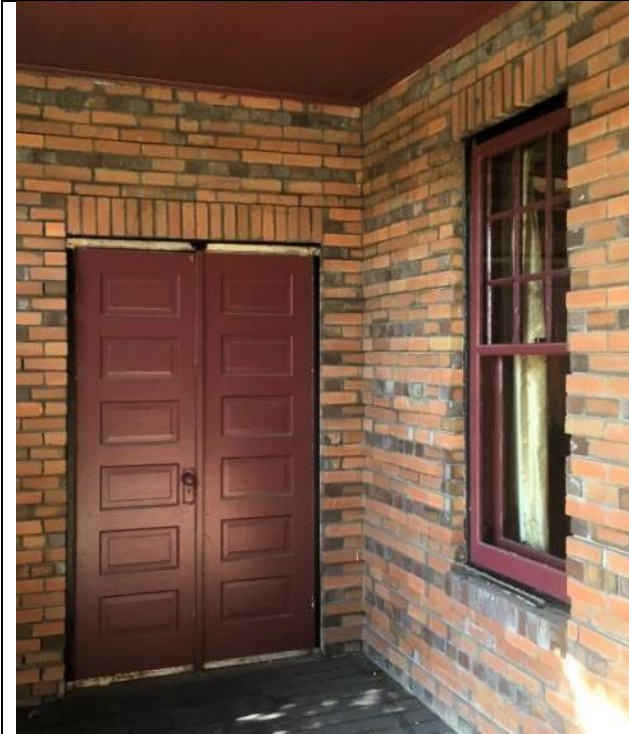
Image 4.2: Example of the paired, six-panel wood doors in the inset central porch (west side).
