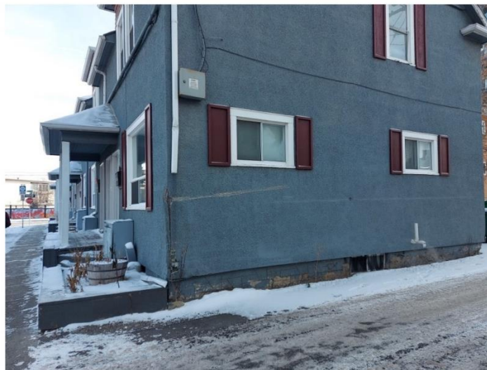
Figure 2: Damage to the northwest corner of the Lunenberg townhouses.
