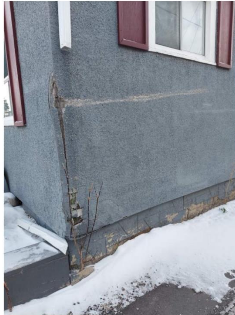
Figure 1: Damage to the northwest corner of the Lunenberg townhouses.
