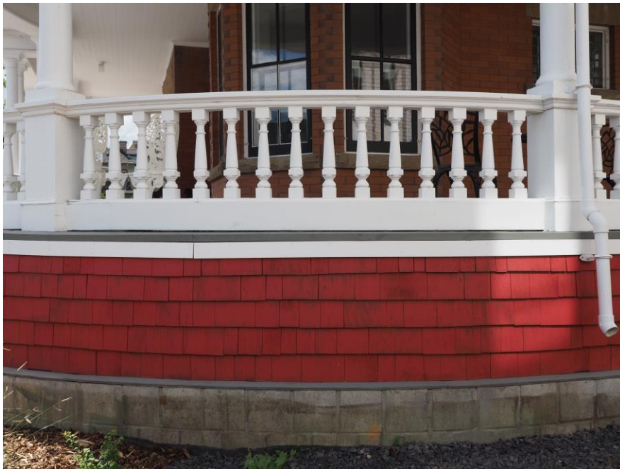
(Image 1.11 – Detail view of veranda skirt at northeast corner of the Nimmons Residence, showing baluster and column profile)
