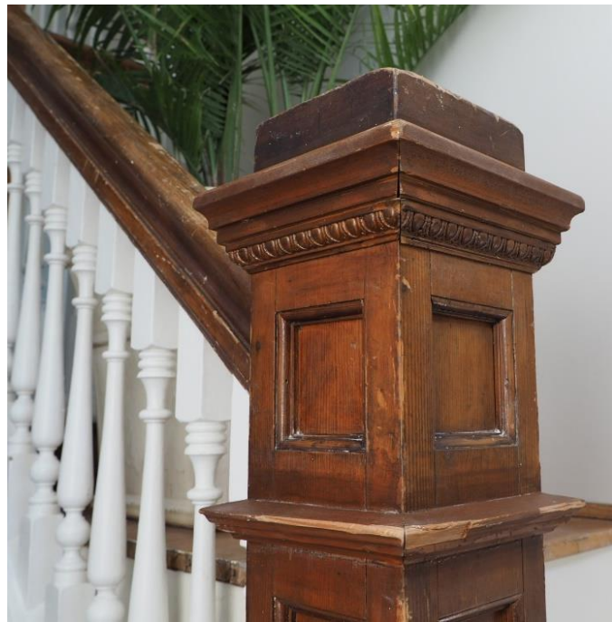
(Image 6.8 – Detail showing newel post at landing between first and second storeys)
