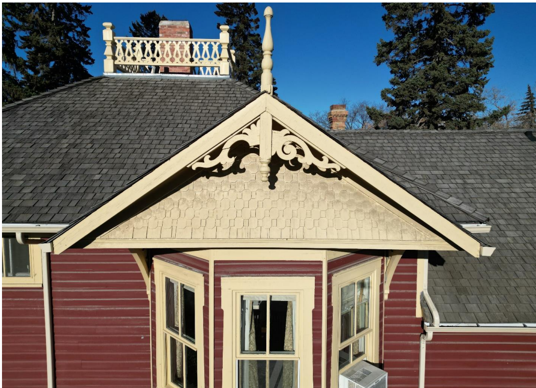
(Image 2.3: Example of one of two projecting two-storey bays with angled gable pediment, clad in wooden octagonal and square shingles, projecting verge with profiled wooden frieze, tongue-and-groove wooden soffits, plain wooden bargeboard, decorative scrollwork and finial, and supported by wooden brackets with decorative panel inlay)
