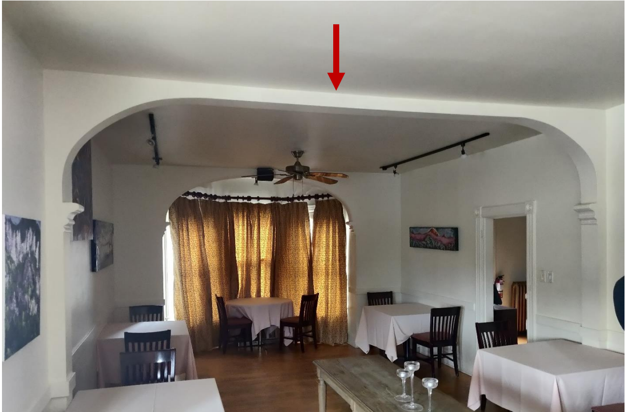
(Image 6.11: Example of central wall curvature in the main room at second level, as denoted with arrow)
