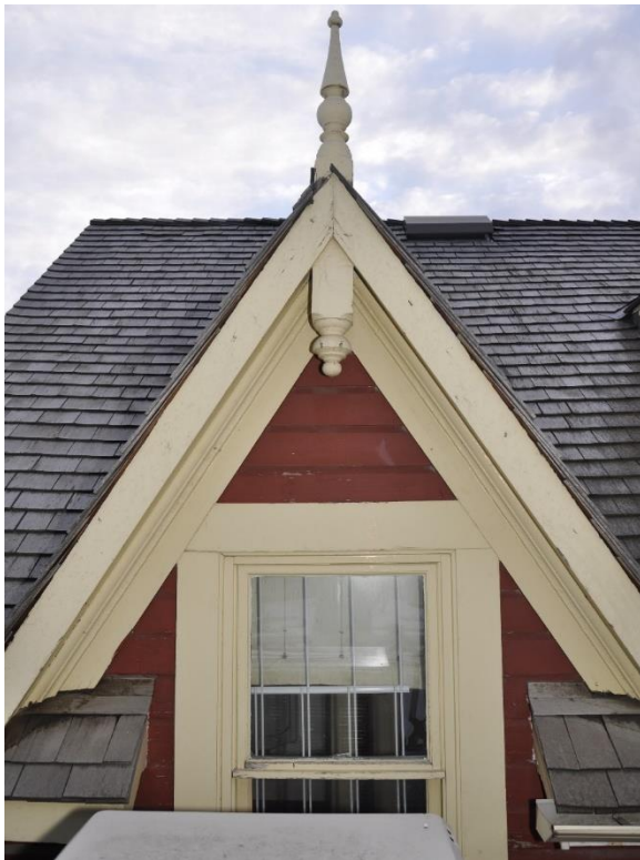
(Image 2.7: West-facing gabled dormer clad in wooden siding, projecting verges with profiled wooden frieze, tongue-and-groove wooden soffits, plain wooden bargeboard, finial)
