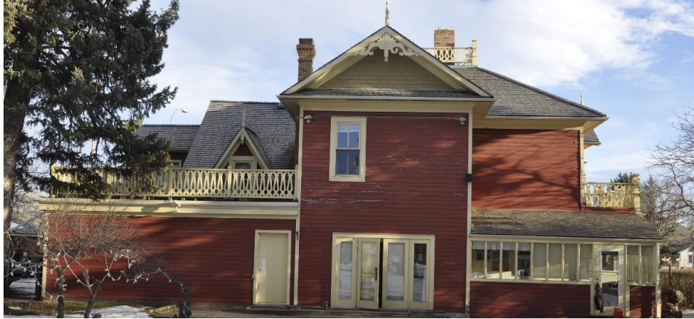
(Image 4.2: Building Section 1 – west façade showing sunroom addition with narrow eaves and projecting two-storey addition with pedimented gable clad in wooden square shingles, projecting verge with profiled wooden frieze, tongue-and-groove wooden soffits, plain wooden bargeboard, decorative scrollwork and finial. Building Section 2 – gabled dormer)
