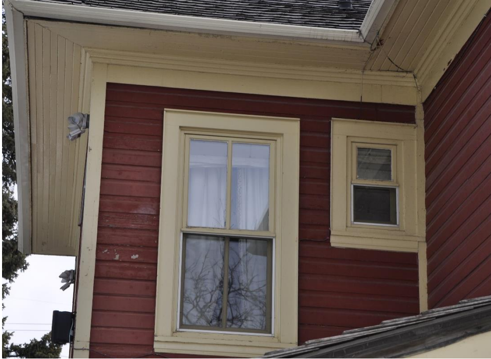
(Image 2.2: Example of overhanging eaves with profiled wooden frieze, plain wooden fascia, tongue-and-groove wooden soffits)
