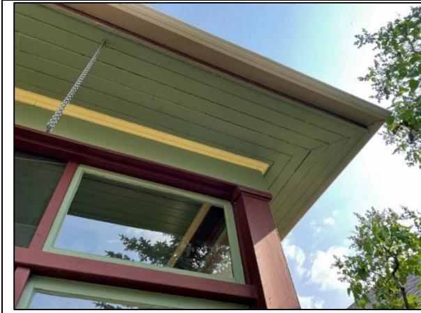
(Image 1.3: Overhanging eaves, wooden tongue-and-groove soffits, moulded wooden frieze, plain wooden fascia)
