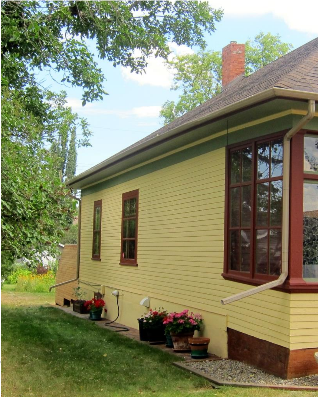
(Image 1.2: North façade showing six-light double-assembly wooden window sashes evenly segmented by wooden mullions, posts, heads and sills (enclosed verandah); 1-over-1 wooden window sash, wooden mullions, heads and sills; beveled-wood siding; moulded frieze, plain wooden fascia, overhanging eaves. Note: storm windows are not regulated)
