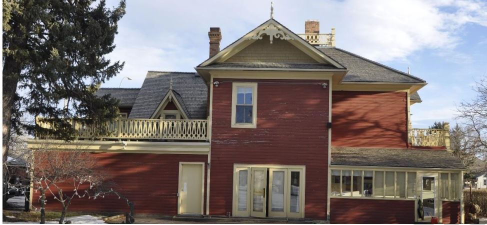
(Image 4.2: Building Section 1 – west façade showing sunroom addition with narrow eaves and projecting two-storey addition with pedimented gable clad in wooden square shingles, projecting verge with profiled wooden frieze, tongue-and-groove wooden soffits, plain wooden bargeboard, decorative scrollwork and finial. Building Section 2 – gabled dormer)
