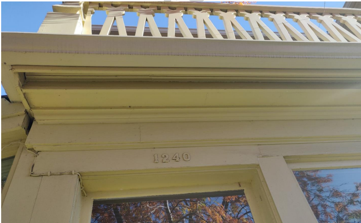
(Image 2.5: South-facing enclosed verandah: eaves, built-up wooden soffit, profiled wooden frieze and plain wooden fascia)
