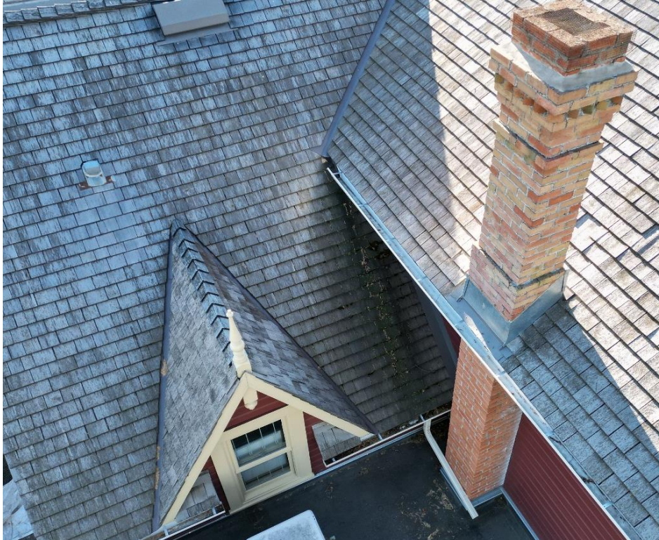
(Image 2.8: Original red brick chimney with heavily corbelled top. West-facing gable dormer with single-hung sash window can also be seen in this photo)
