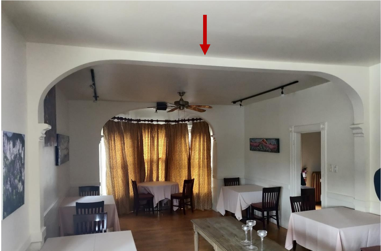
(Image 6.11: Example of central wall curvature in the main room at second level, as denoted with arrow)
