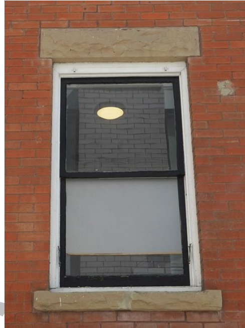
(Image 1.4 – Example of a typical 1-over-1 wooden-sash window; sandstone lintel above the window opening and sill below)
