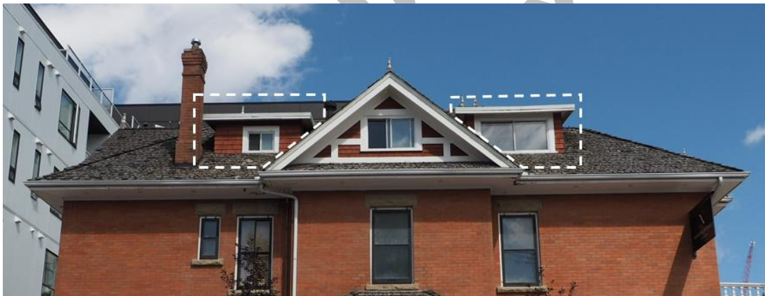
(Image 5.2 – Upper floor & roof detail of south façade; non-regulated shed-roof dormers indicated with dotted outline)
