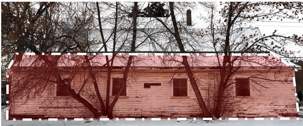
(Image 5.1: North façade; shed-roof addition indicated in red shading and outlined in white dash-dotted line is not regulated)
