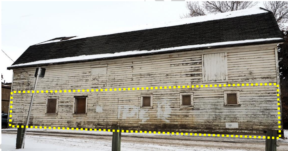
(Image 3.2: South façade; fenestration and existing windows on the first story as outlined in dotted lines are not regulated)
