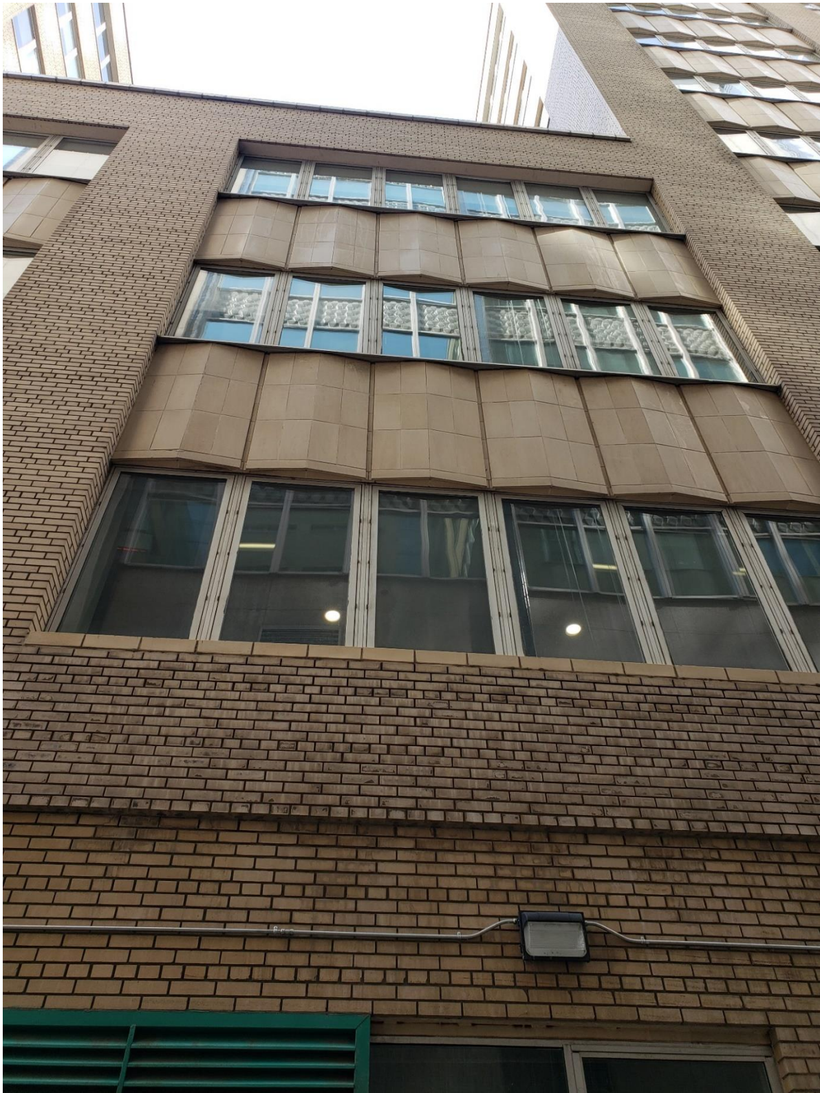
(Image 3.7: Detail view of buff-coloured brick cladding in common bond and angled 'chevron' glazed terra cotta tile spandrel panels, north façade)
