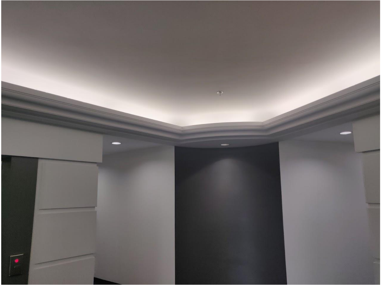
(Image 4.2: third floor elevator lobby, wall curvature)
