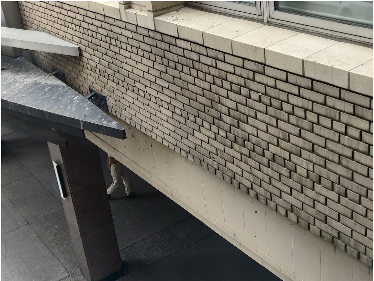
(Image 3.9: Detail view showing a granite column, glazed moulded terra cotta signband, buff-coloured brick cladding, and terra cotta sills on second storey)
