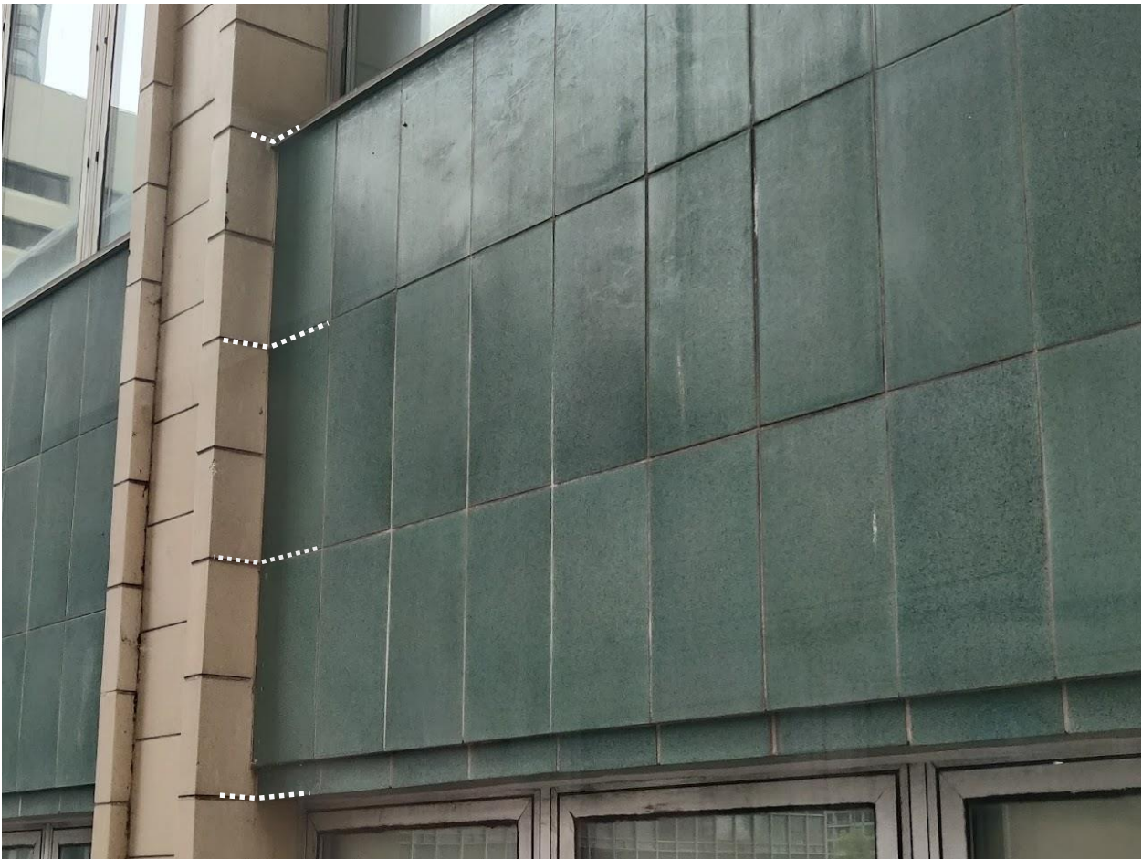
(Image 3.6: Glazed green tile spandrel panels set into structural grid with matching mortar joints between spandrels and pilasters, as denoted with white dotted lines)
