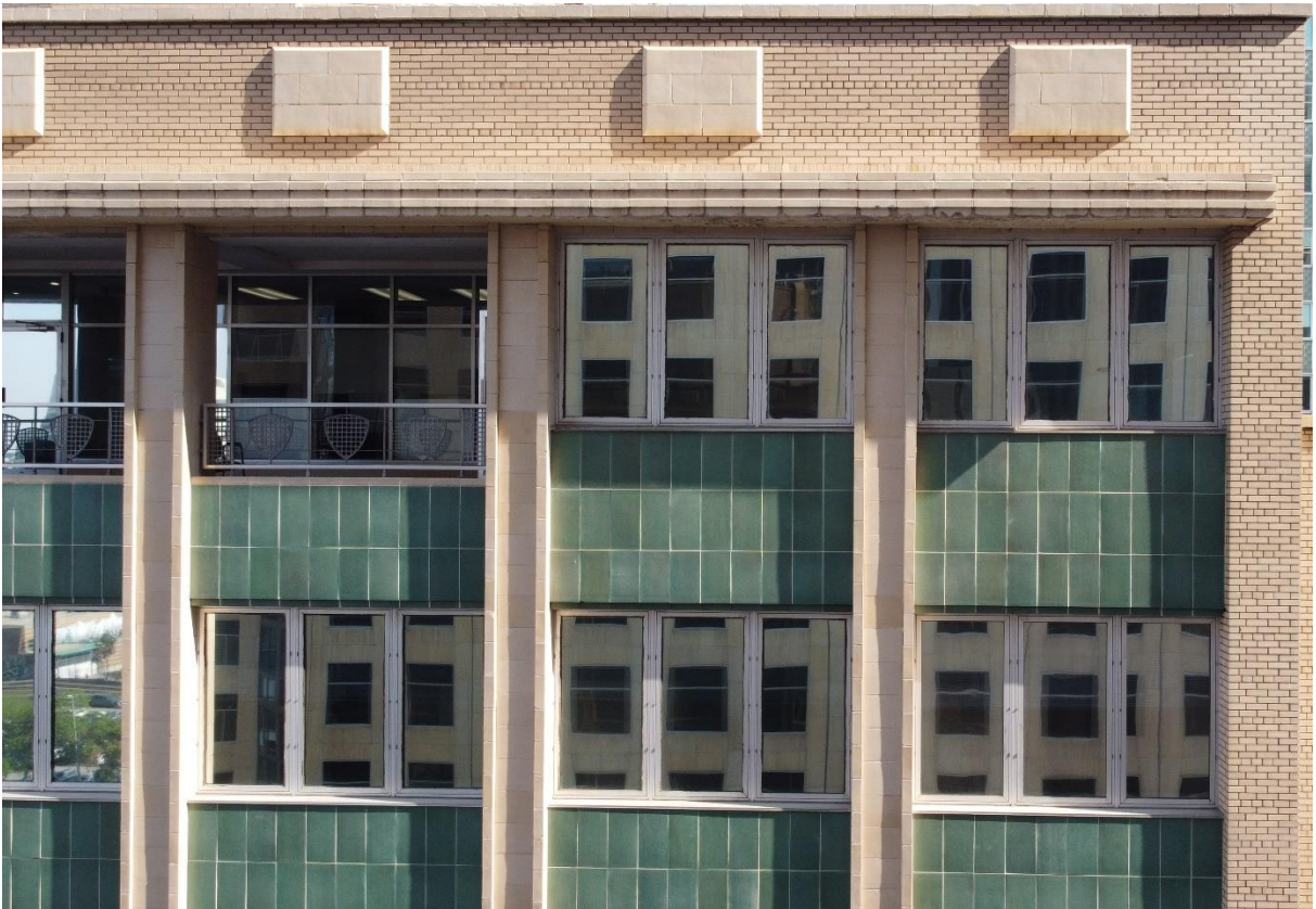
(Image 2.1: Parapet with glazed terra cotta coping, relief stone panels with projecting moulded canopy beneath – south façade)
