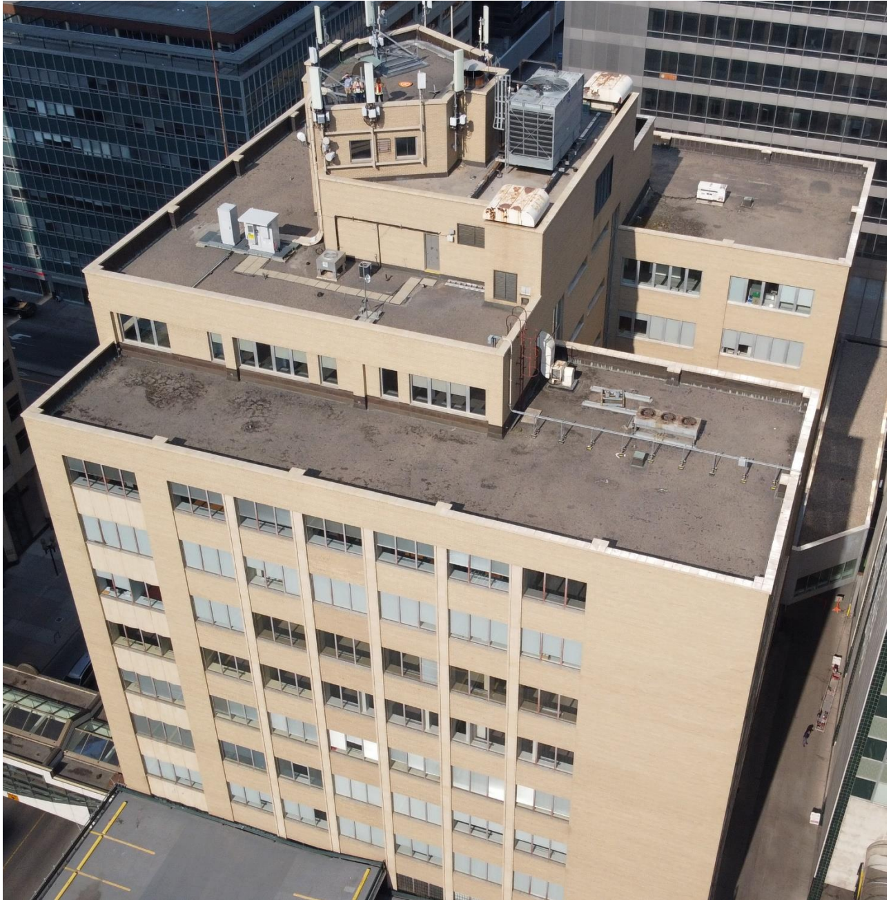
(Image 3.4: Aerial view of east façade and portions of north façade, north façade fenestration including repeating five-pane vertical window sash pattern, rooftop penthouse, elevator and mechanical structure)
