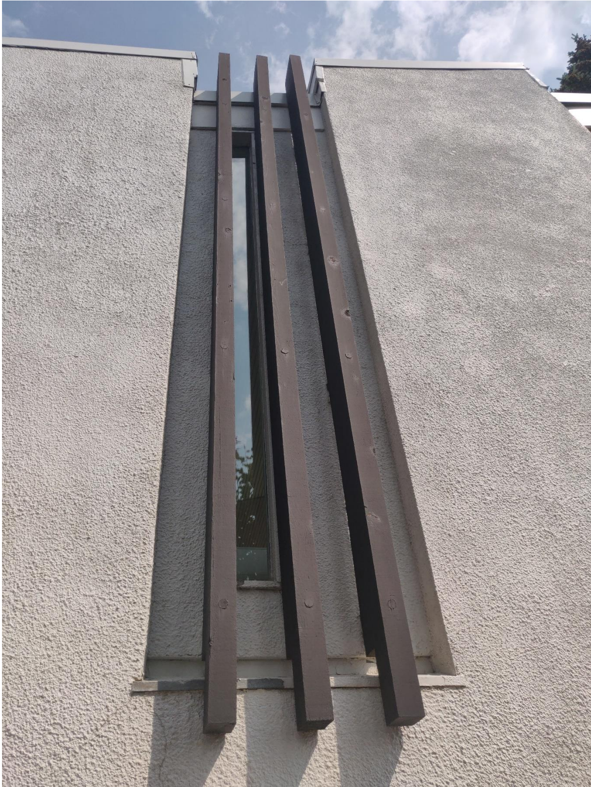
(Image 5.3: Recessed wall with tall narrow window slit and three projecting vertically-oriented wood slats)
