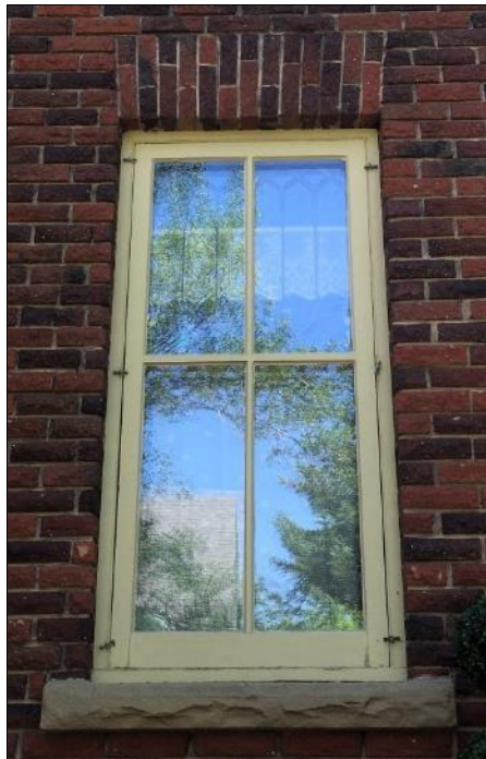
Image 6.5: Example of original fenestration, a beveled leaded glass-over-single-pane window, jack brick arch header and sandstone sill. Note: Storm window in place over window.
