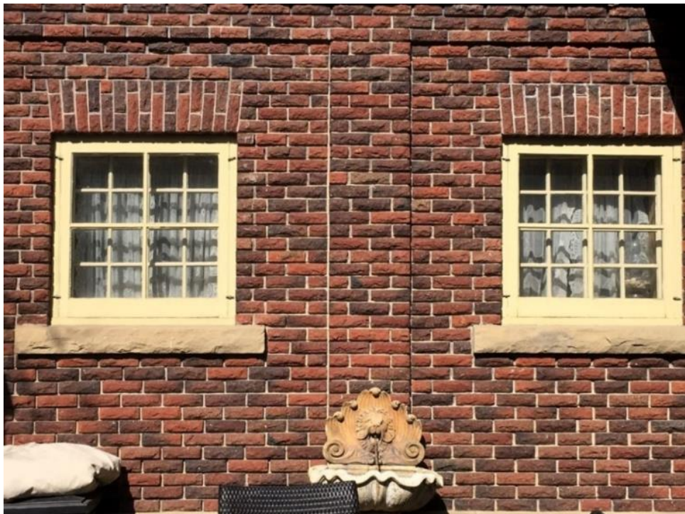
(Image 6.3: Detail of recessed brick panels on rear garage extension and original fenestration of multi-pane glass windows, jack arch brick headers and sandstone sills. Note: Storm windows in place over windows)
