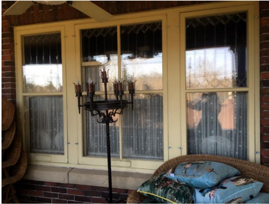
(Images 3.7: Example a triple window assembly, wood mullins, jack brick arch header and sandstone sill. Note: Storm windows in place over windows)
