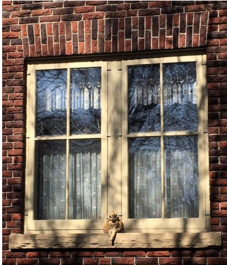
(Image 4.7: Detail of original fenestration, a paired assembly of multi-pane, beveled leaded glass-over-single pane windows, wood mullion, jack brick arch header and sandstone still. Note: Storm windows in place over windows.)
