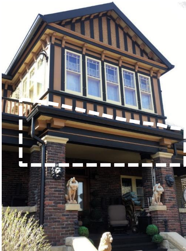
(Image 3.6: Southeast façade oblique image close up. The area demarked with white dashed lines details how the jettied sunroom rests on the projecting ends of the jetty joists above the paired sandstone capitals)
