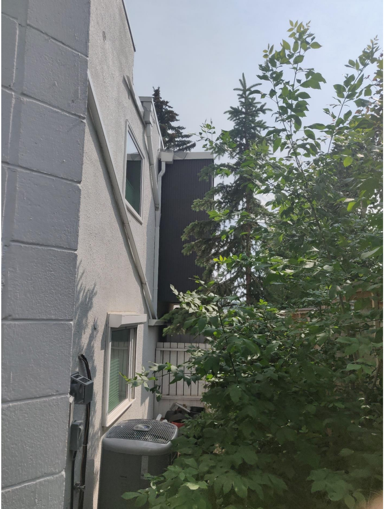
(Image 5.2: Oblique view of west façade showing the cantilevered bump-out from the north-west corner)
