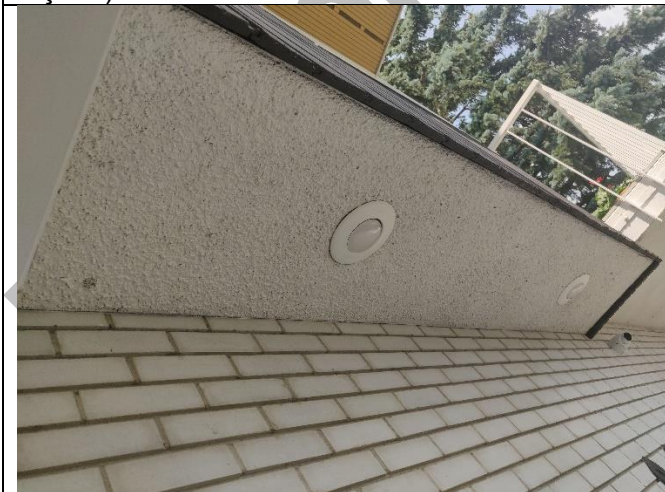
(Image 2.3: Potlights located beneath bump-out on south façade)
