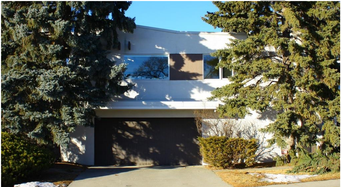
(Image 4.1: East façade, 2011. Flush garage entrance and awning, exposed wooden beam ends)
