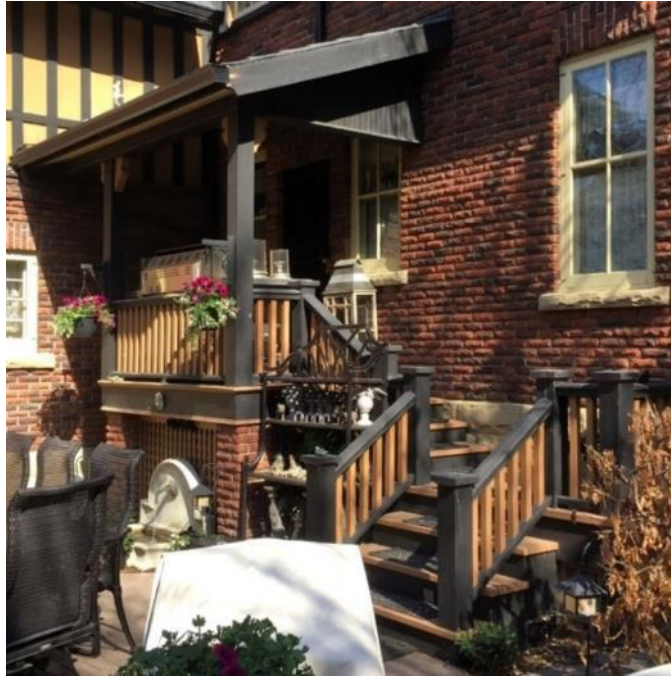
(Image 6.4: Detail of porch, shed roof, wood hand rail, posts, balustrade and brick piers)
