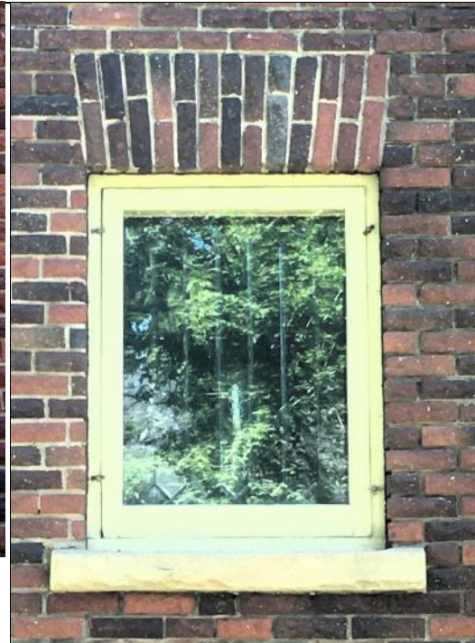
Image 5.5: Example of original fenestration, a fixed, multi-pane, beveled, leaded glass window. Note: Storm window in place over window.
