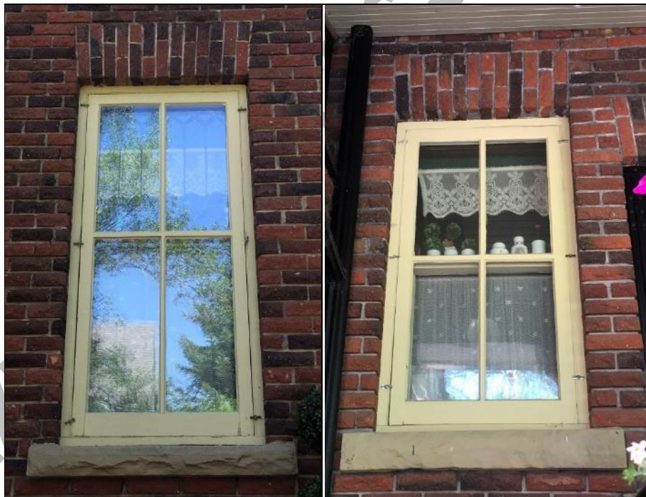
Image 6.5: Example of original fenestration, a beveled leaded glass-over-single-pane window, jack brick arch header and sandstone sill. Note: Storm window in place over window.
