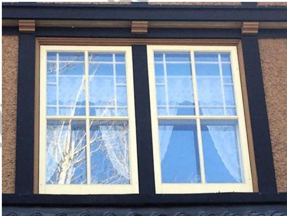
(Image 5.6: Example of original fenestration, a paired assembly of multi-pane-glass-over-single pane windows, wood mullion and wood sill. Note: Storm windows in place over windows)
