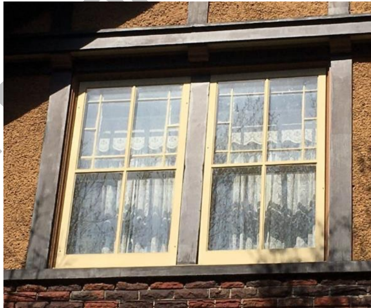
(Image 4.8: Detail of original fenestration, a paired assembly of multi-pane-glass-over-single pane windows, wood mullion and wood sill. Note: Storm windows in place over windows.)
