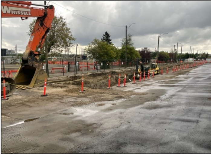
EAST BELTLINE - Deep utility relocation work along 12 Avenue S.E., east of 5 Street S.E.
