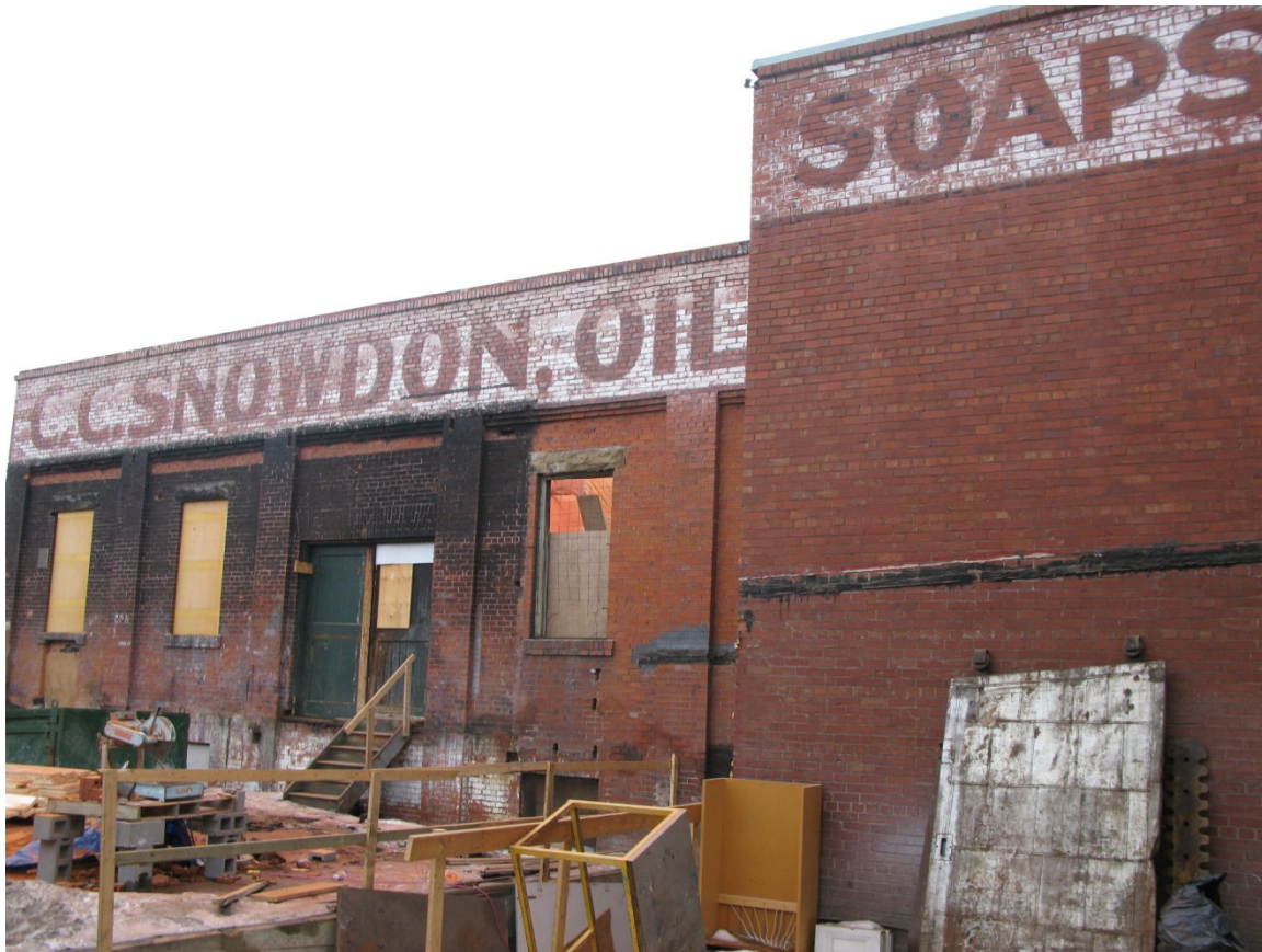
(Photo 5.3: Easterly portion of North Façade showing 1911 building section, left, and a rear extension to the 1913-14 building section, added in the 1910s or 1920s)
