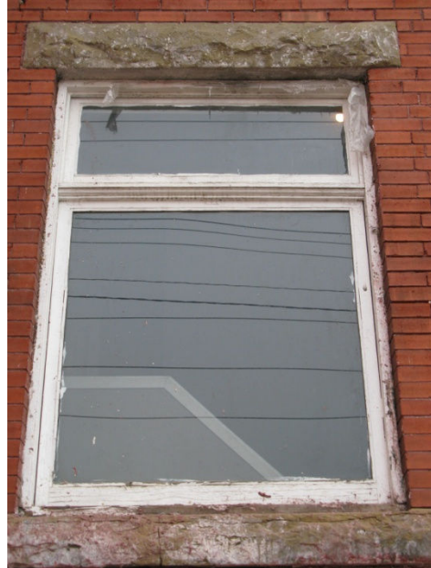
(Photo 2.7: an example of a wooden-sash window with a single-light hopper transom over a fixed, single-light sash of the 1911 building section – shows sandstone sill and lintel)
