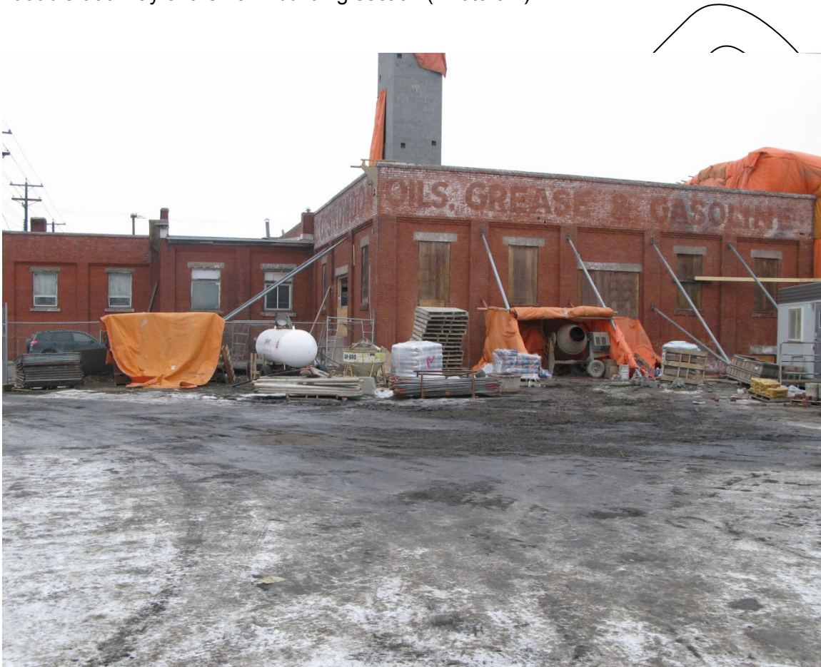
(Photo 3.2.) South Façade. Note- photo shows site during construction of new rooftop addition with new elevator shaft rising above the historic roofline.)
