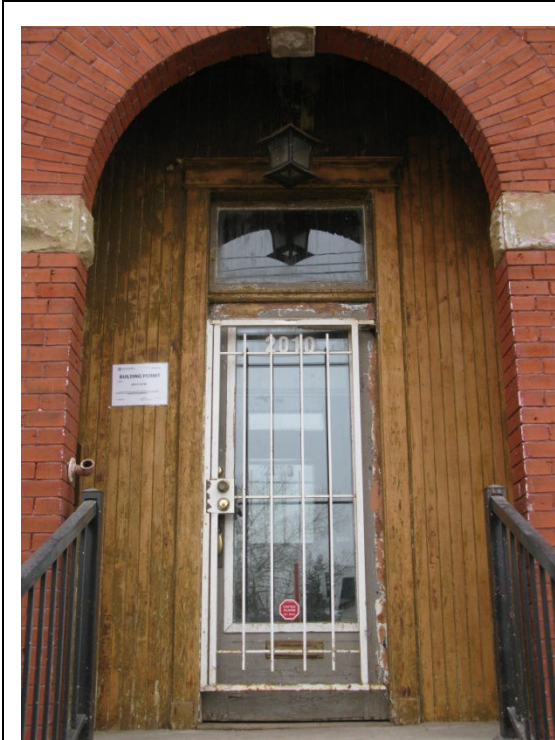
(Photo 2.10: central doorway of the 1911 building section with inset, wooden, tongue-and-groove assembly wall containing a single door with transom light and wood casings.)
