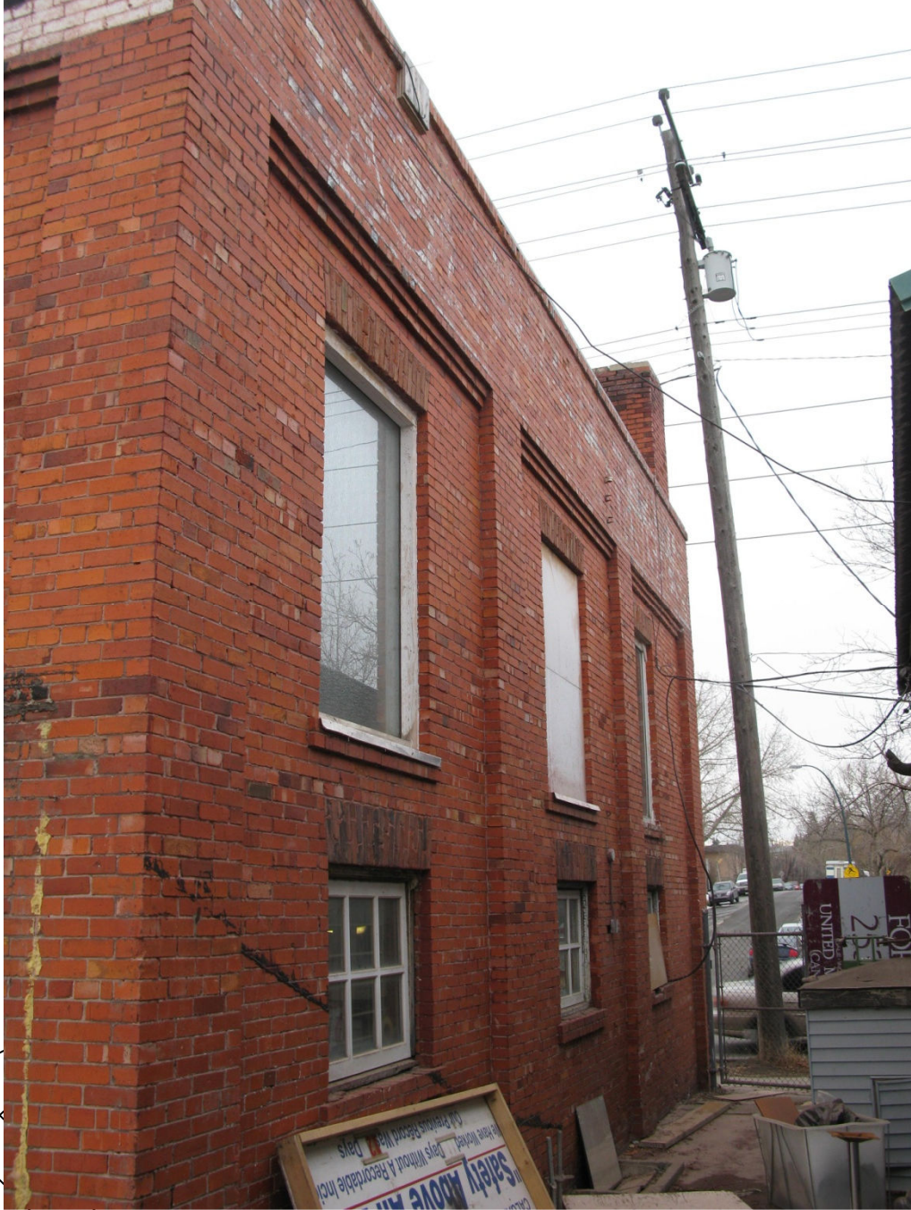
(Photo 5.4: oblique view of Westerly portion of North Façade showing 1913-14 building section)
