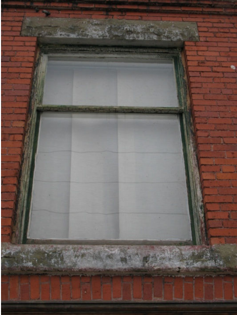
(Photo 2.6: an example of a wooden, one-over-one, hung-sash windows of the 1913-14 building section – shows sandstone sill and lintel)
