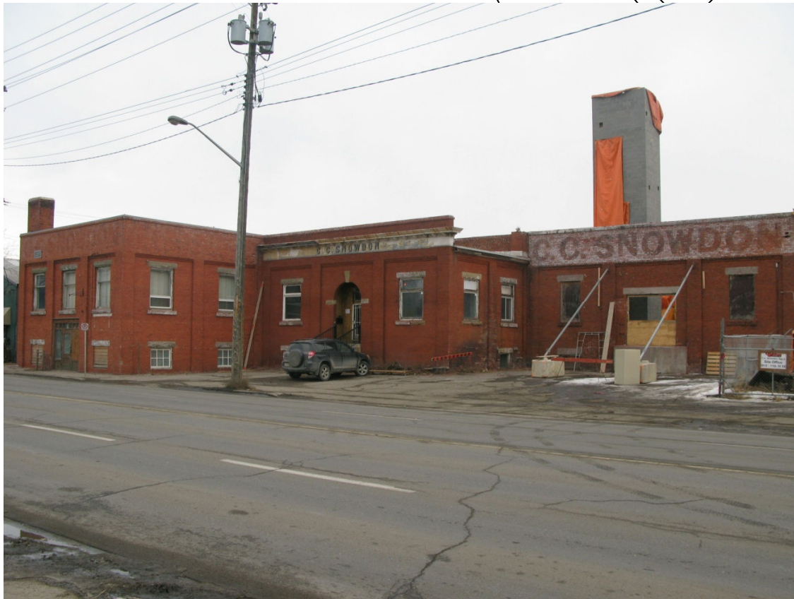
(Photo 2.2: oblique view from the southwest of the West Façade. Note- photo shows site during construction of new rooftop addition with new elevator shaft rising above the historic roofline.)
