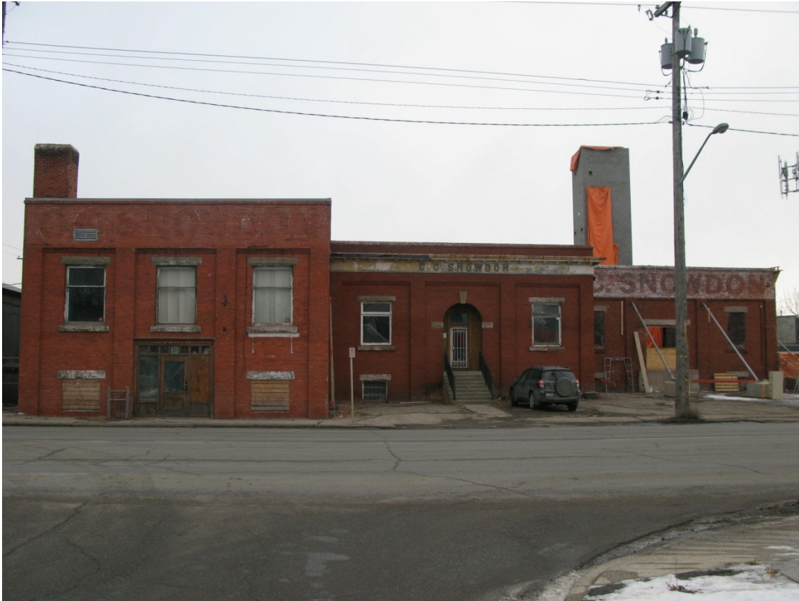
(Photo 2.3: West Façade. Note photo shows site during construction of new rooftop addition with new elevator shaft rising above the historic roofline.)
