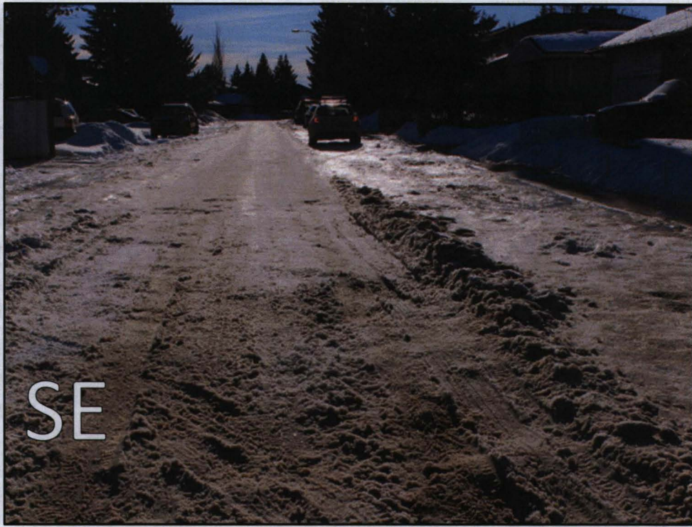
A snow covered road that was flat bladed down the centre in the southeast.
