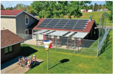
ABOVE The new solar panels at the Glenbrook Community Association in Southwest Calgary.
