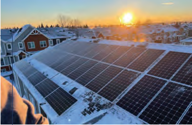
ABOVE The latest solar installation supported by ENMAX. REACH at Martindale is a 12-building multi-family development with an arrangement of regular and stacked townhomes and includes 116 residential homes.
