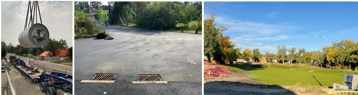
FROM L TO R: UPPER PLATEAU SEPARATION, NWIC LOCAL IMPROVEMENTS ON SUNNYHILL LANE, TUXEDO PARK DRY POND.
