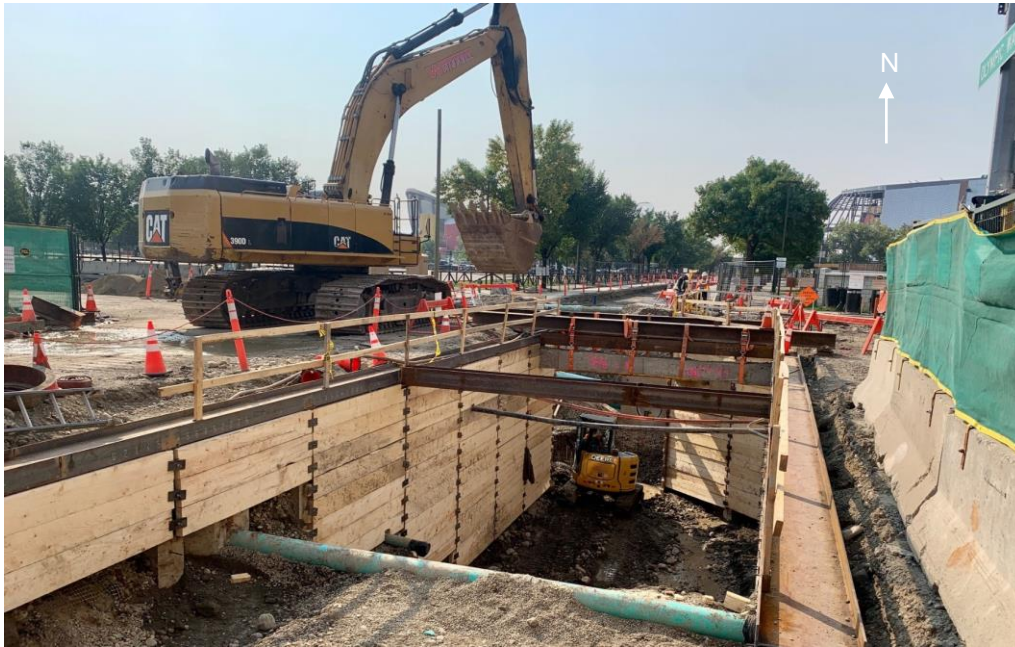
Sanitary and Storm trunk works at the intersection of Olympic Way and 12 Ave SE
