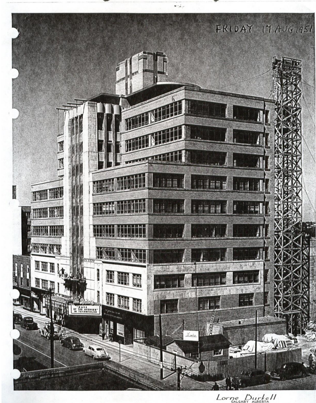
(Image 1.2: 1951 photo showing oblique view of south façade with deep overhanging eaves at the eleventh storey penthouse, and original rooftop mechanical and elevator house forms, geometric-patterned stone banding on elevator house at the rooftop). Photo Credit: Daniel Barron
