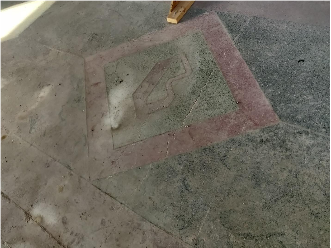
(Image 5.2: Detailed view of terrazzo flooring with brass inlay and 'B' formed in the centre of elevator lobbies from floors two through five, and seven through ten, including re-created sixth storey terrazzo floor )
