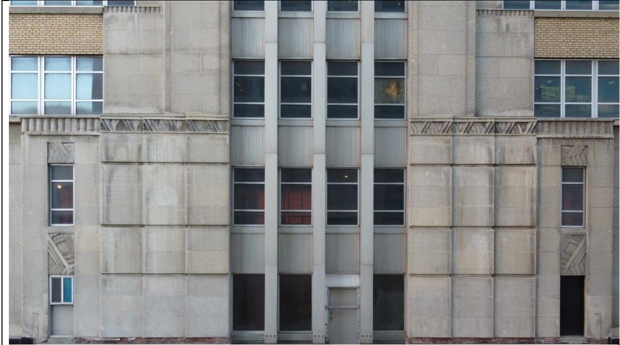
(Image 1.12: Frontal view of carved detail bands and Art Deco motifs on Tyndall limestone)
