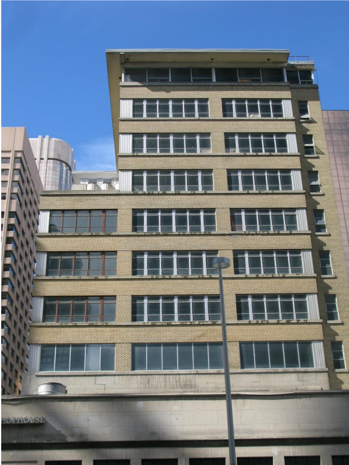
(Image 3.1: View of east façade flat roofs (terraces) where the building steps back at the eighth and eleventh storeys, with deep overhanging eaves at the eleventh storey penthouse, and original rooftop mechanical and elevator house forms, buff-coloured brick spandrel panels framing storeys four through eight)
