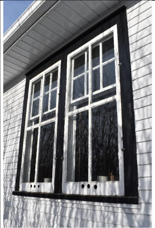
2.11: Detail of typical fenestration, paired assembly, wood frames and narrow plain lug wood sill.
