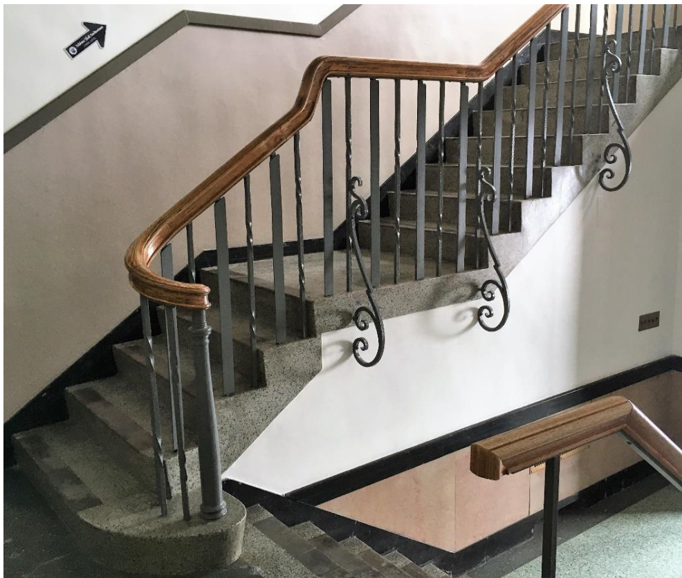
(Image 3.3: Lower portion of double return main staircase, cast-iron newel post, ornamental wrought iron balustrade and decorative bracket supports)
