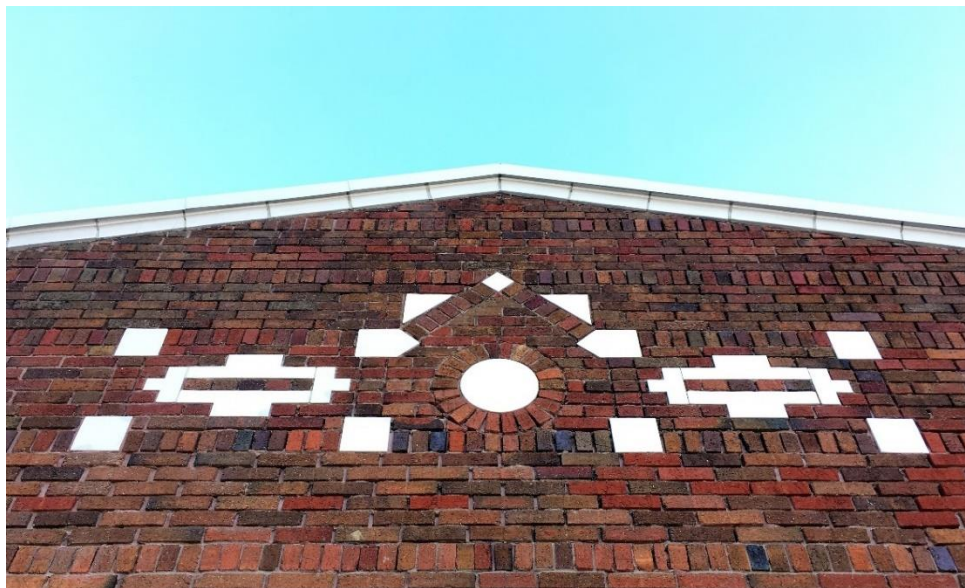
(Image 1.3: Detail of triangular pediment with terra cotta coping and inlaid tiles)
