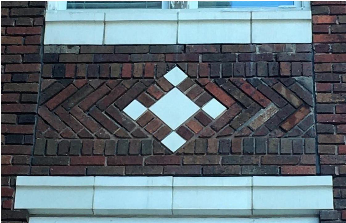
(Image 1.6: Herringbone brick pattern with inlaid terra cotta tiles, lintels and sills)
