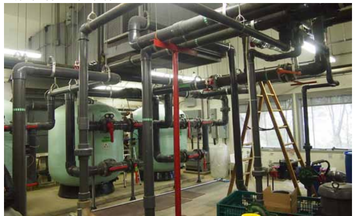
Pool mechanical room
