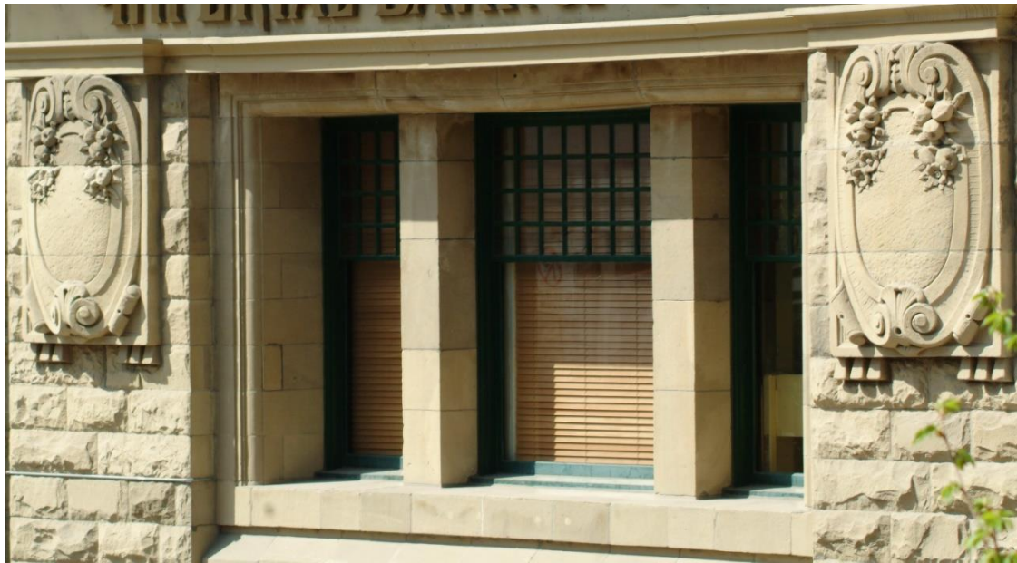
(Image 1.8: Detail of triple assembly window, deep moulded window surround, sandstone mullions)
