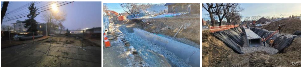
TUXEDO COMMUNITY DRAINAINGE IMPROVEMENTS, FROM L TO R: 18 AVENUE NE TRUNK DIVERSION, 35 AVENUE NE TRUNK UPGRADE, TUXEDO PARK DRY POND.
