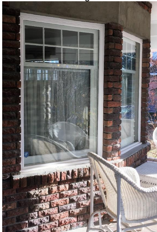
(Image 2.4: Detail of bow window; concrete headers; brick lintels; painted wood window casings)
