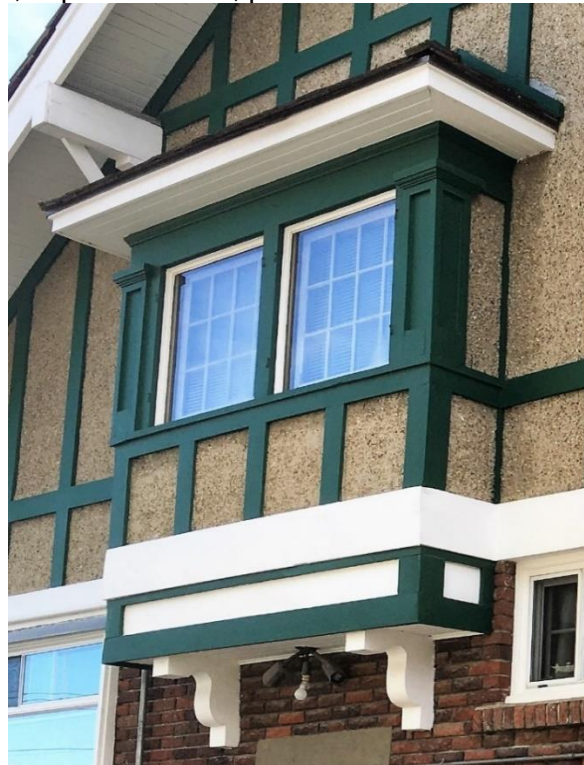
(Image 2.10: Detail of box bay window; hip roof; deep tongue-and-groove eaves; painted wood casing and moulded brackets)
