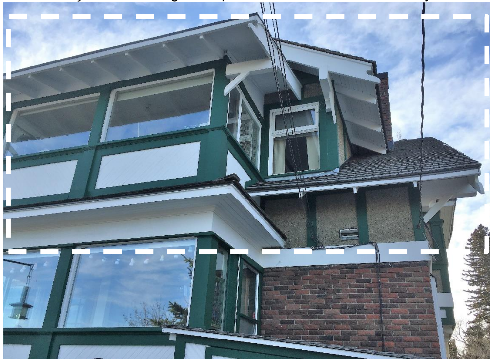
(Image 2.15: Rear façade. Note. Regulated portions are in area demarked by the dashed line))
