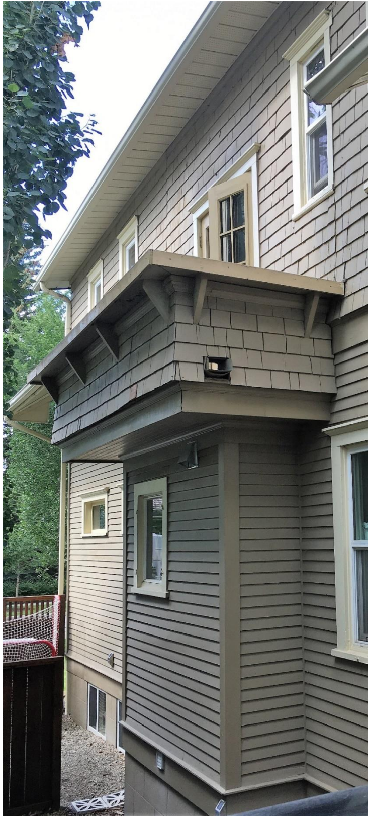
(Image 2.6: Detail of three-sided bay, upper level balcony with wood shingle cladding, closed balustrade; wood moulding and fascia; tongue-and-groove soffit)
