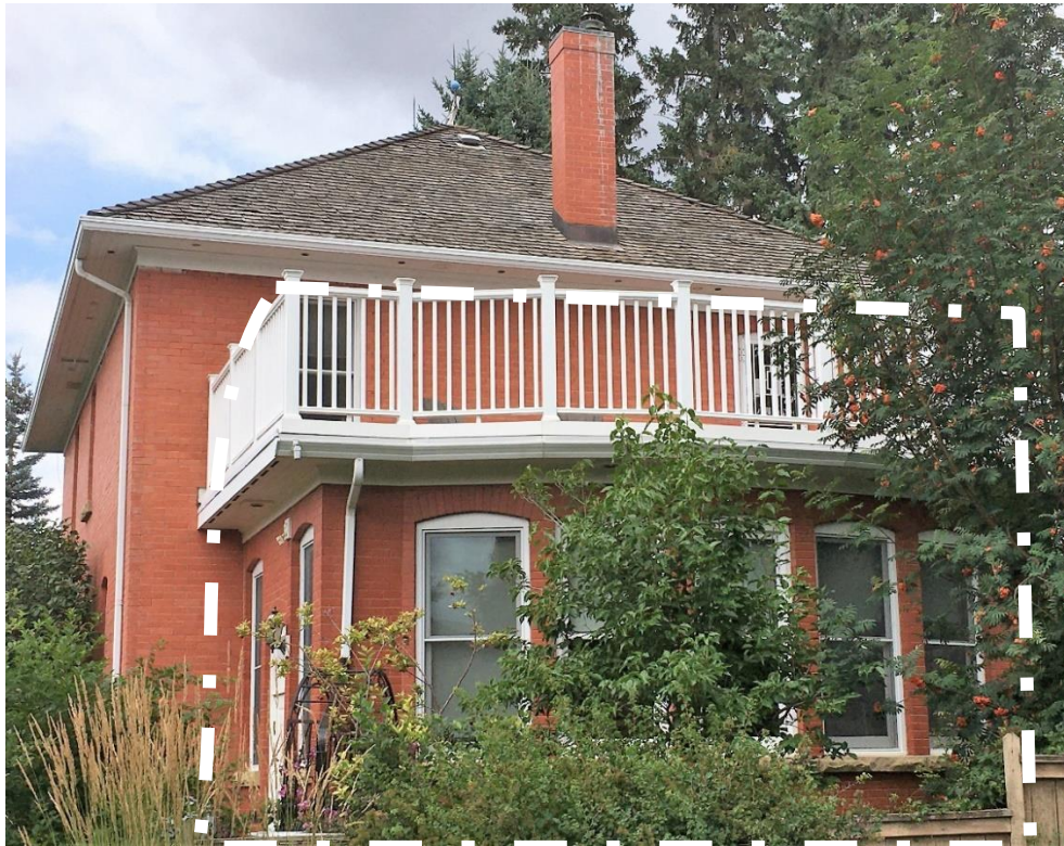
(Image 2.7: South façade. Note: White dashed line delineates unregulated portions (main floor addition and upper balcony))
