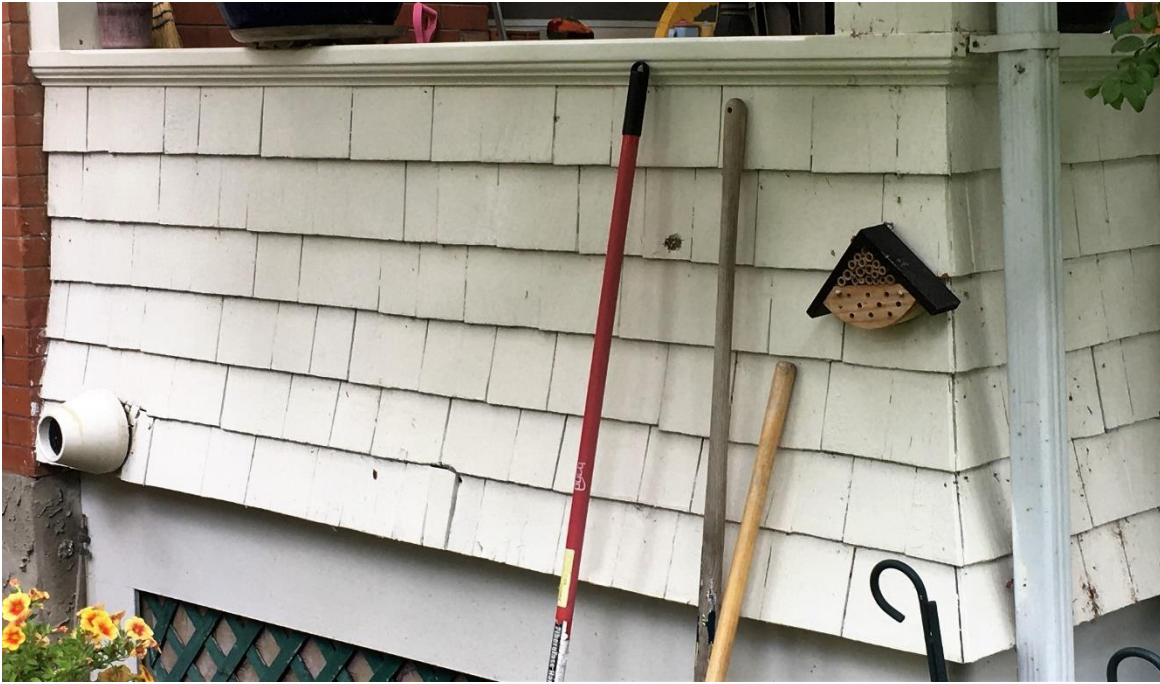
(Image 2.4: Detail of wood shingle clad verandah with flared, wood shingle corners)
