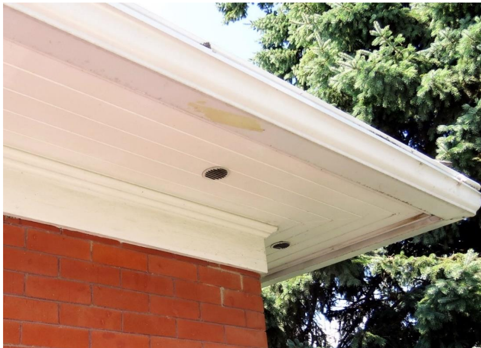
(Image 3.2: Detail of eave; wooden tongue-and-groove soffits, wooden fascia and moulded frieze)
