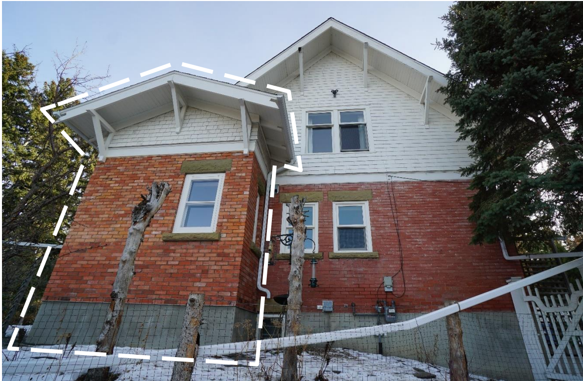
(Image 2.2: Northwest façade. Dashed outline indicates the corner single storey extension built ca. 2013 that, while sympathetically designed, is not regulated)
