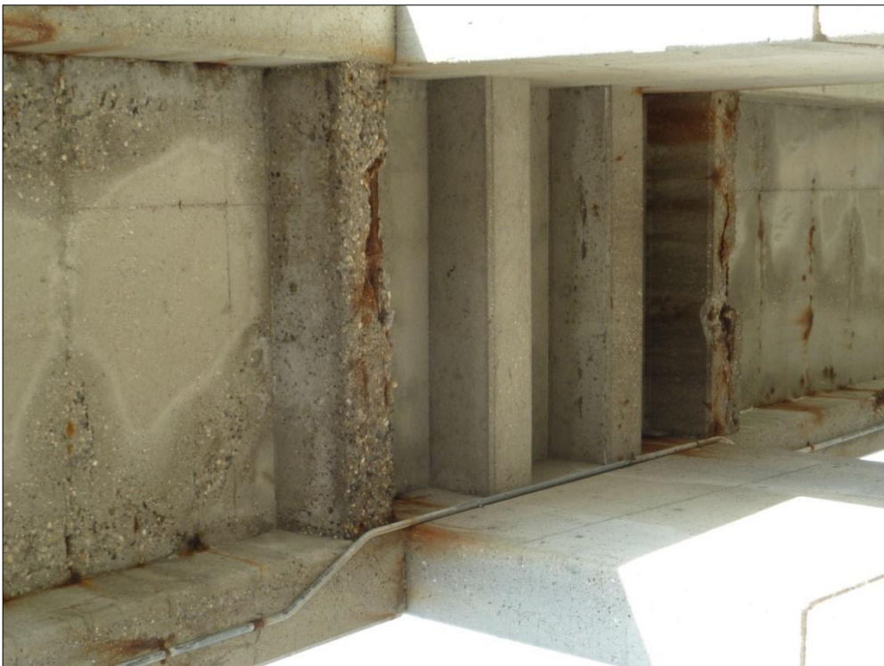
Figure 8: East Ramp Soffit -Spalling of concrete, rebar exposed
