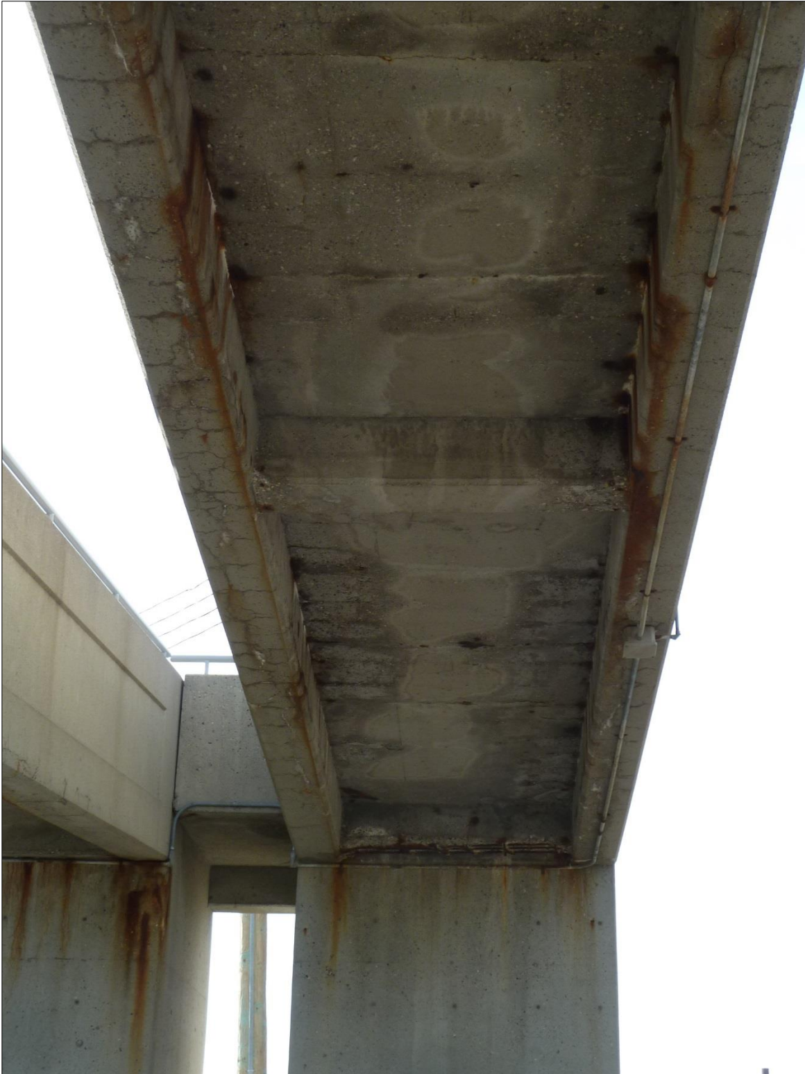
Figure 11: East Ramp Soffit - Longitudinal and transverse cracks, exposed rebar on diaphragm
