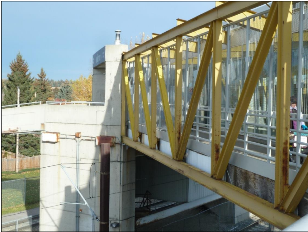
Figure 13: Paint peeling off on steel truss
