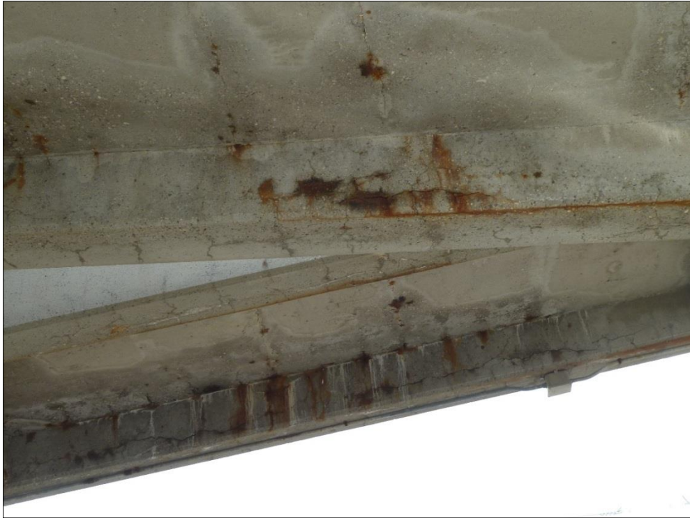
Figure 12: East Ramp Soffit - Longitudinal and transverse cracks with rust stains
