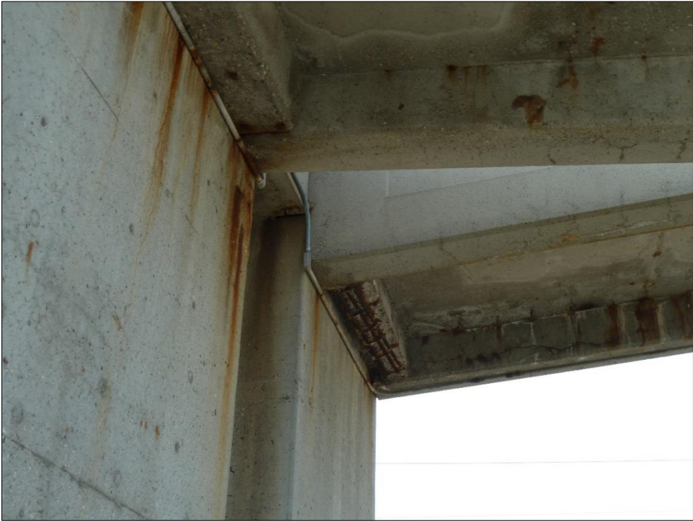
Figure 9: East Ramp Pier -Rebar exposed on diaphragm, rust stains
