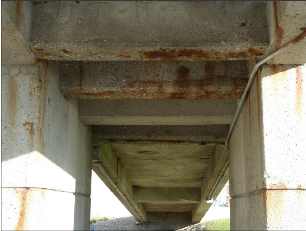
Figure 7: East Ramp Soffit - Longitudinal cracks, rust stains
