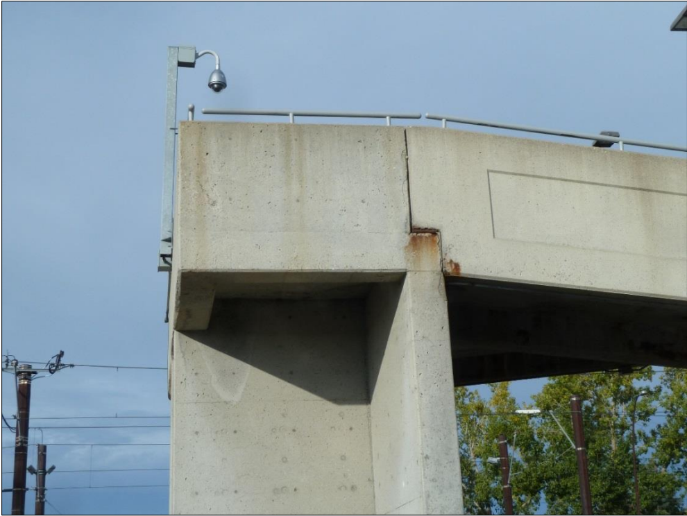
Figure 10: East Ramp Pier - Rust stains
